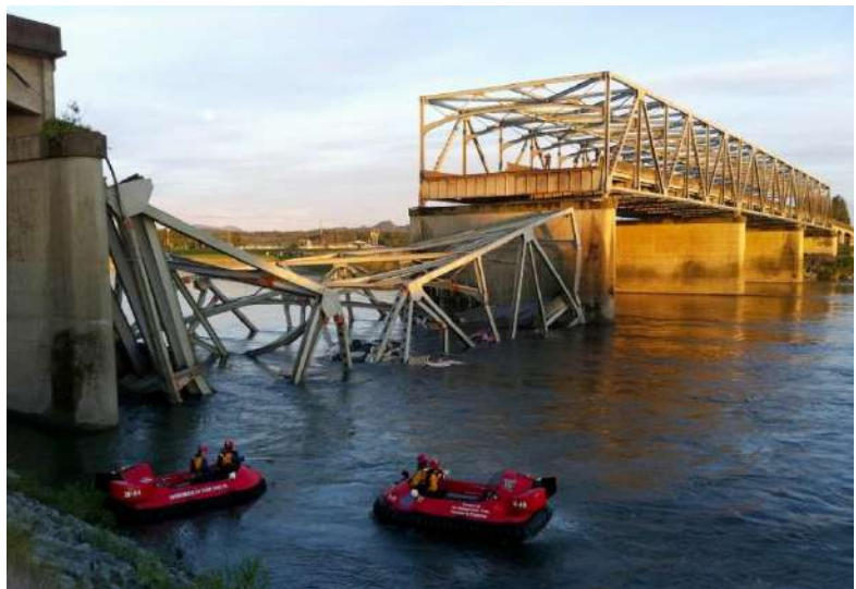
Figure 3-8 Skagit County Bridge Collapse
