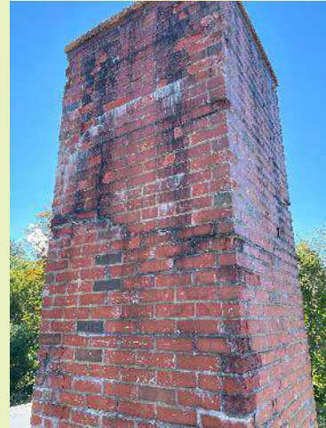
Maple Avenue Elementary Chimney Condition
