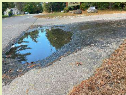
Glen Lake School Roadway Entrance Pooling
