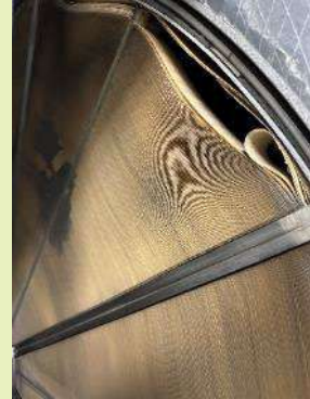
Bartlett Elementary School ERV-1 Energy Wheel
