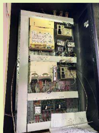
Bartlett Elementary School Boiler Room Controller
