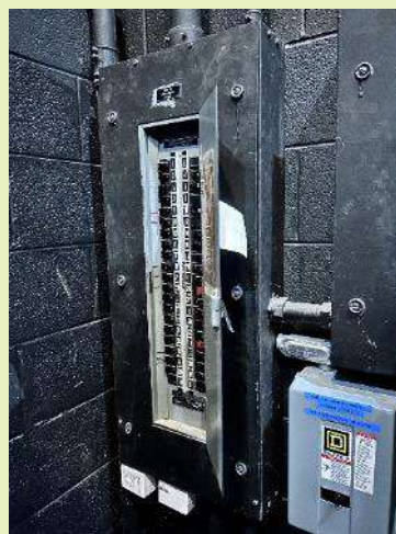
Goffstown High School Electrical Distribution Panel
