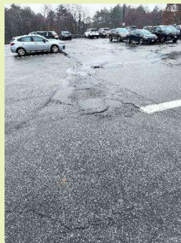
Mountain View Middle School Parking Lot Deterioration
