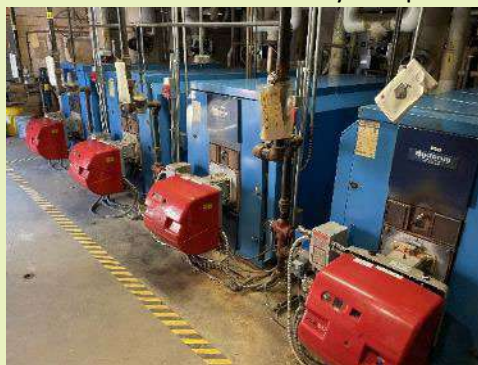
Goffstown High School Boiler System
