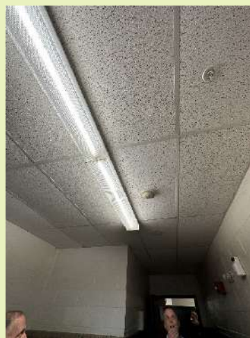
Bartlett Elementary T8 Lighting
