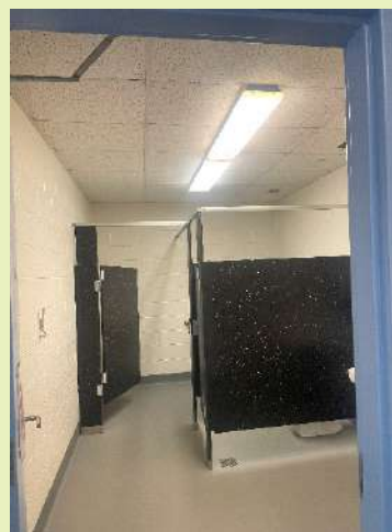
Maple Avenue Elementary T8 Lighting in Bathroom
