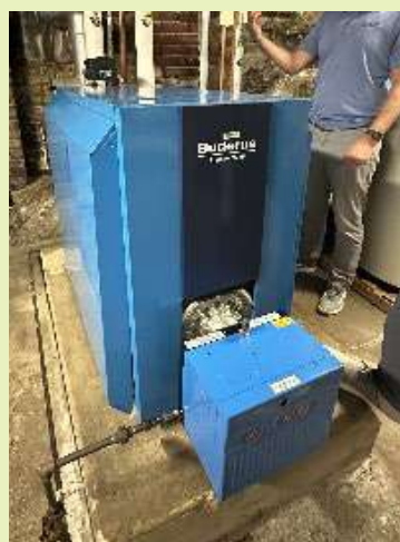
SAU Office Boiler
