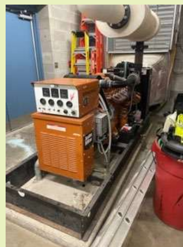
Mountain View Middle School Generator
