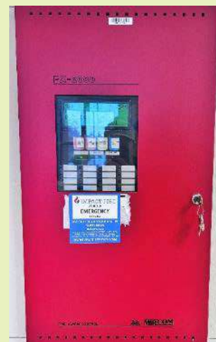
Mountain View Middle School Fire Alarm Panel
