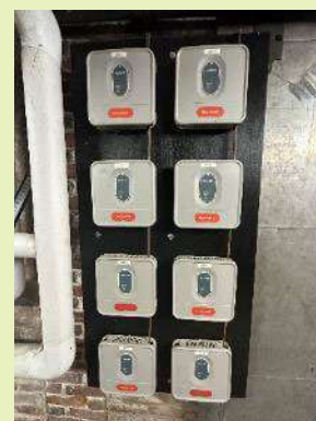
SAU Office Controls
