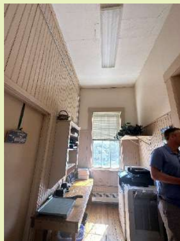
SAU Office T8 Lighting
