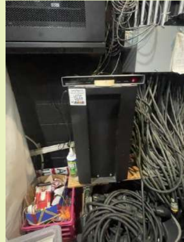
Goffstown High School Lighting Controller
