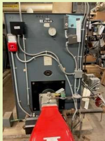
Mountain View Middle School Boiler
