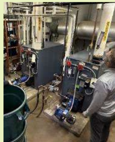
Bartlett Elementary School Boilers
