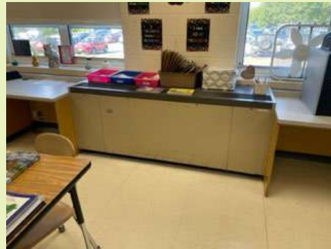
Mountain View Middle School Classroom Unit Ventilators
