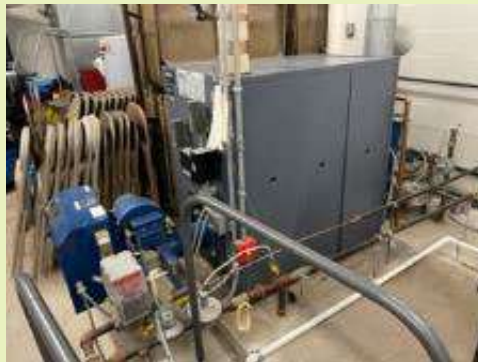
Glen Lake School Aging Boiler
