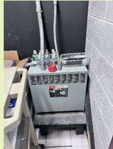
Goffstown High School Building Transformer
