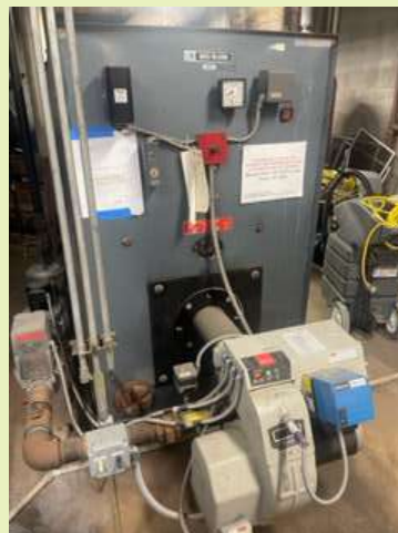
Maple Avenue Elementary Aging Boiler
