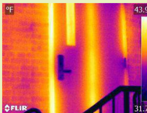
Bartlett Elementary Exterior Door Heat Loss
