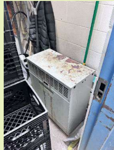
Mountain View Middle School Building Transformer
