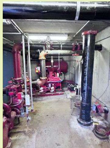
Mountain View Middle School Fire Pump House
