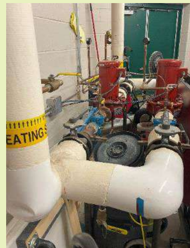
Glen Lake School Hot Water Pumps
