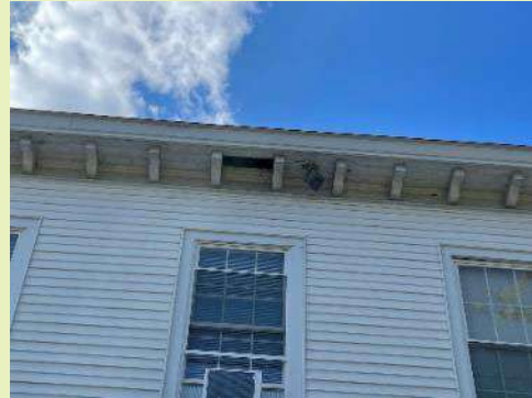
SAU Office Hole in Soffit
