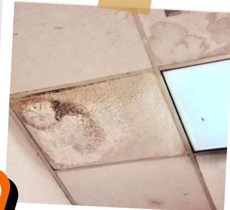
Replace ceiling tiles
