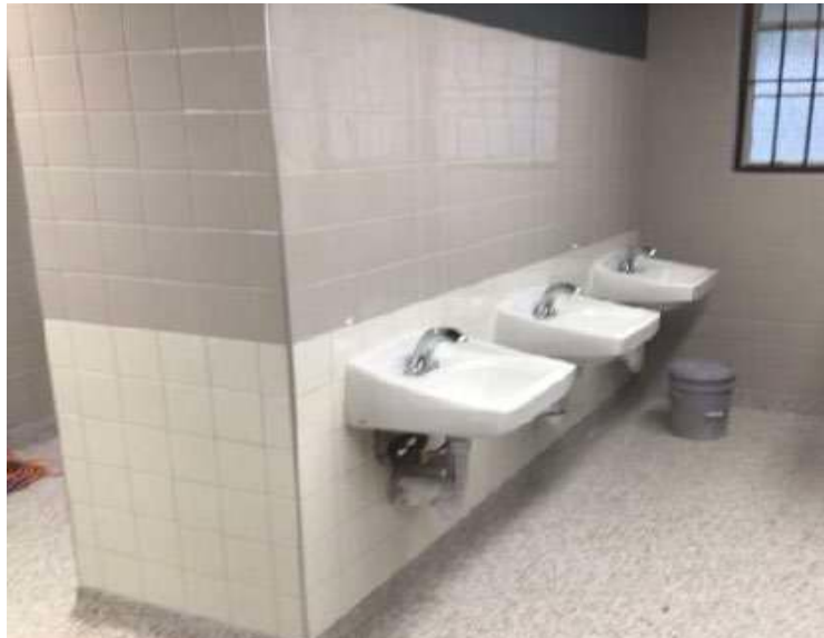
Sinks Installed in Boys' and Girls' Restrooms
