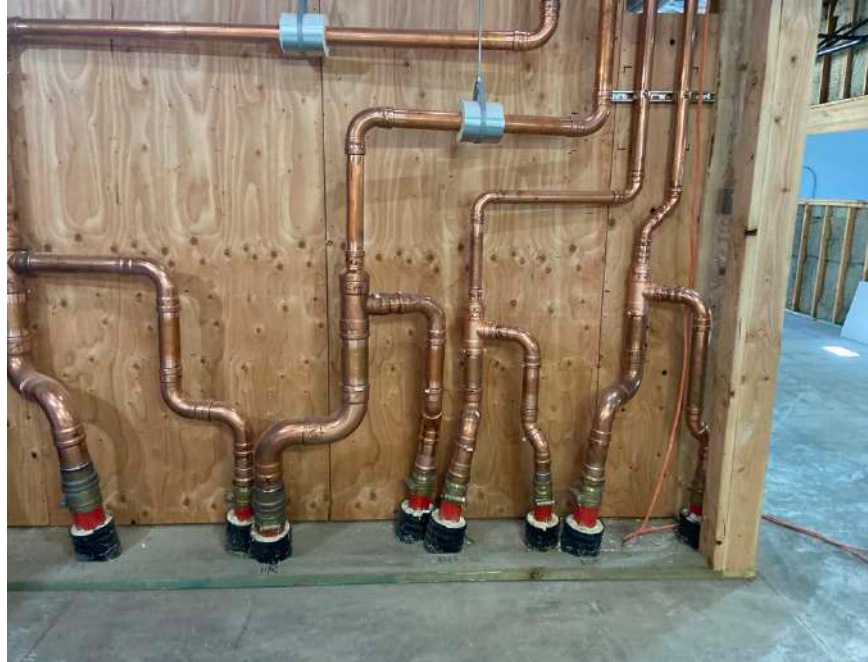
NEW HYDRONIC LINES AT THE NEW BUILDING
