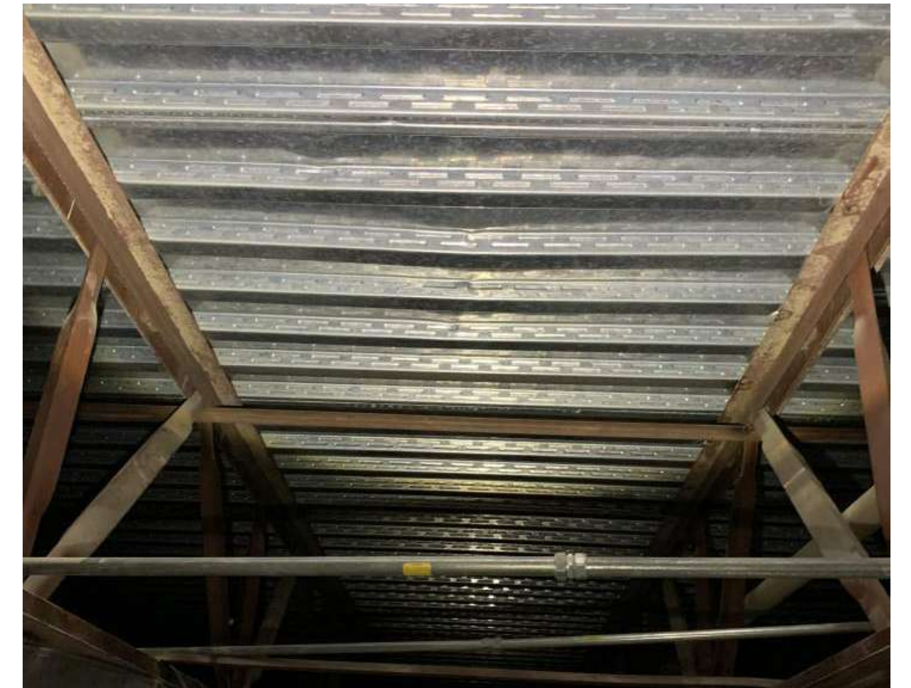
Figure 6. Deformed Metal Deck Below Weight Room (1985 Addition)
