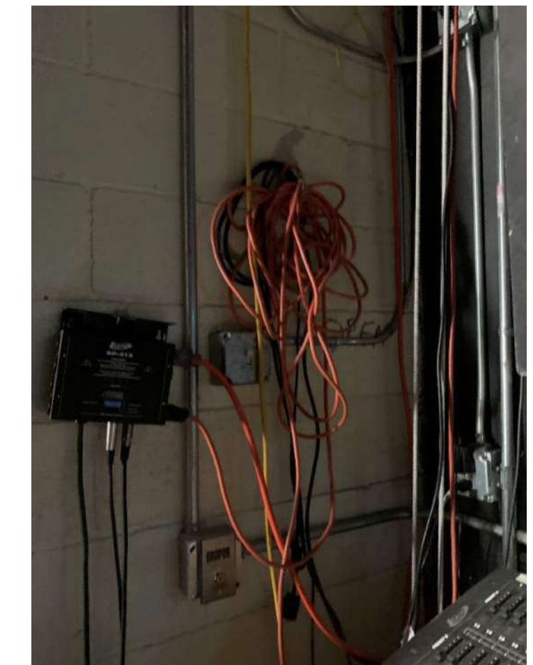
E7: Extension cords at stage area.
