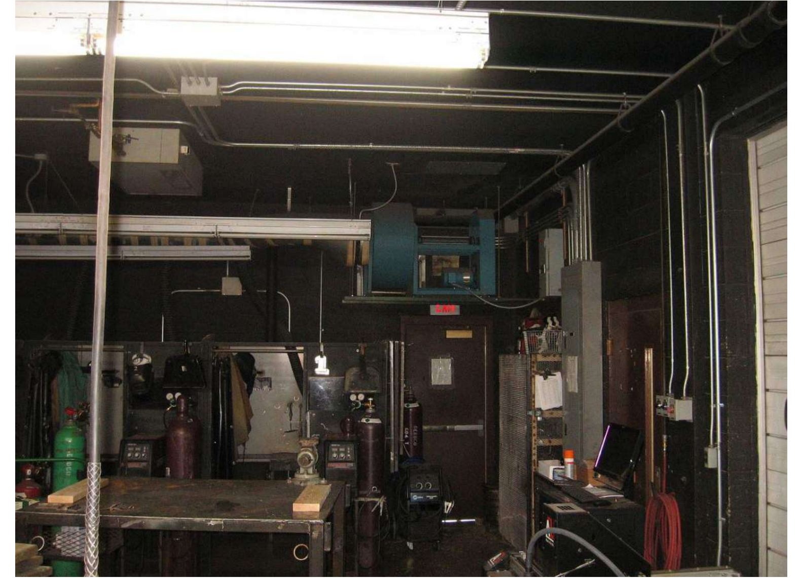
M21: Welding Shop Exhaust Fan
