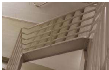
Non-compliant guards at stair
