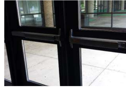
Code compliant panic hardware
