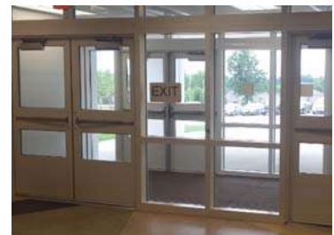
Compliant "EXIT" signage
