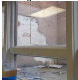
Wall finish delamination
