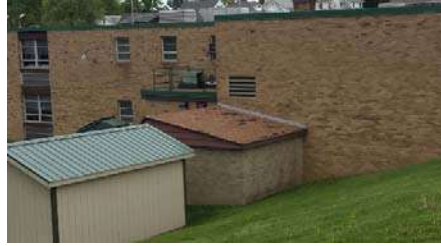
Shingles need replaced
