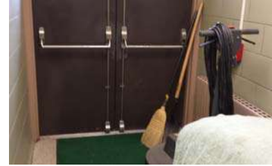
Egress doors blocked
