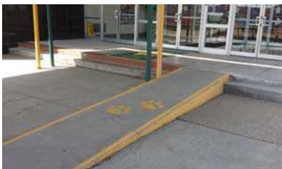
Main entry ramp – no handrails
