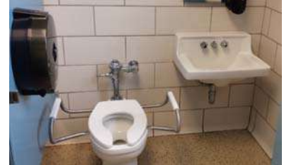
Non-compliant toilet stall
