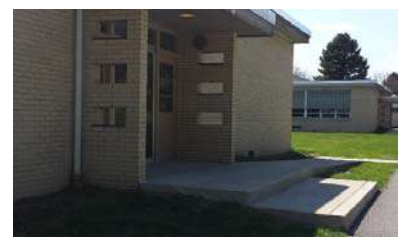
Non accessible – no handrails
