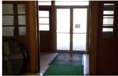
No accessible signage at doors
