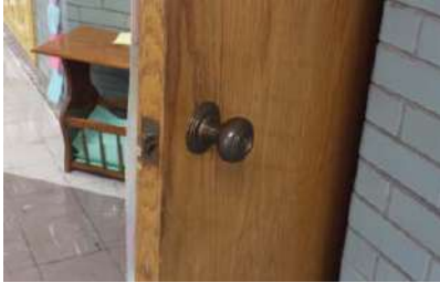
Non accessible door hardware
