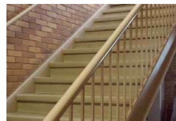
Compliant guards at stair
