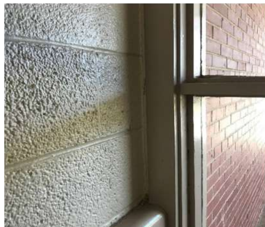
Photo #4 HA# B 16 – Interior Window Caulk
