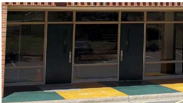
Photo #3 HA# I 21 – Fire Doors (multiple types)
