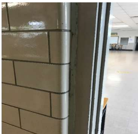
Photo #3 HA# E 10 – Interior Door Caulk
