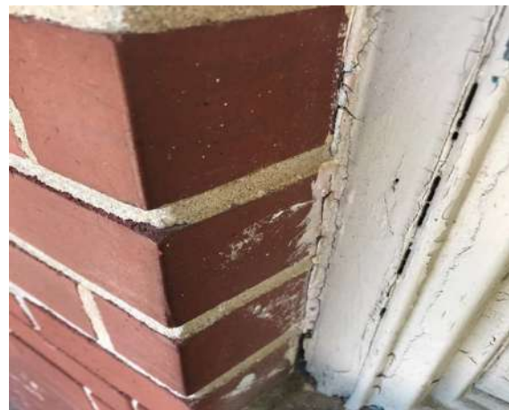
Photo #4 HA# C 8 – Exterior Window Caulk
