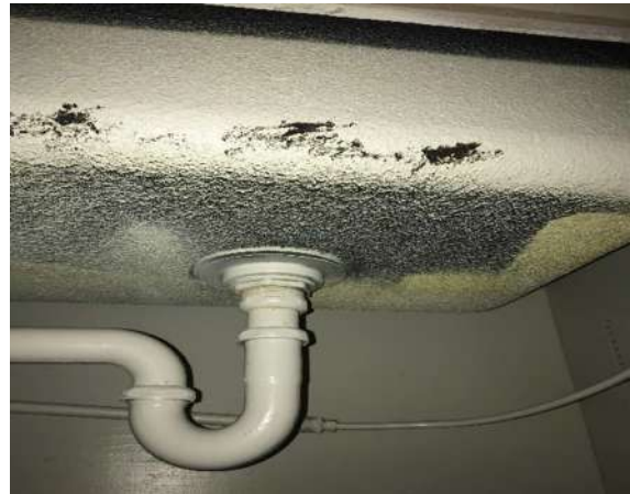
Photo #4 HA# A 17 – White Sink Mastic
