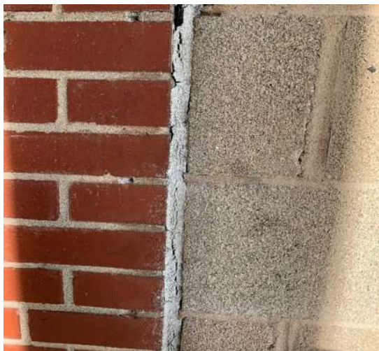
Photo #5 HA# B 19 – White Door Caulk
