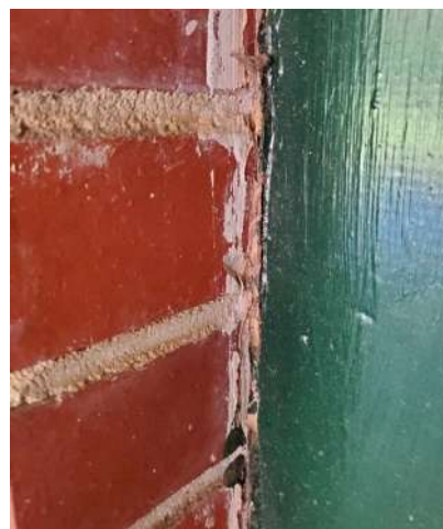
Photo #2 HA# E 9 – White Exterior Door Caulk
