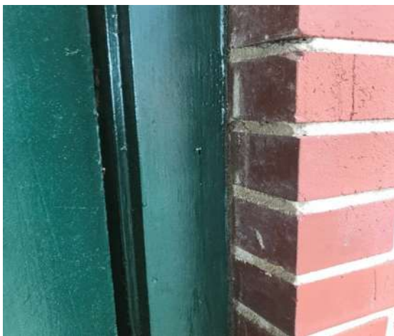
Photo #3 HA# D 8 – Exterior Door Caulk
