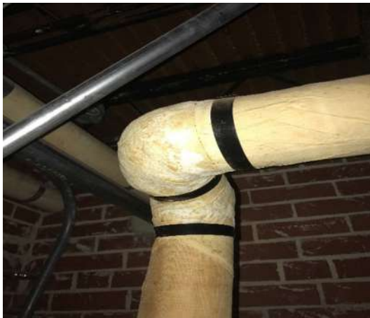
Photo #3 # A 15 – 1" Pipe Elbow Insulation
