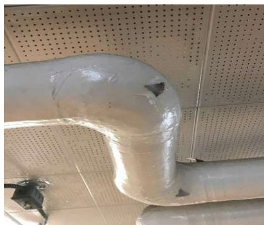
Photo #4 HA# E 11 – 2" Pipe Elbow Insulation
