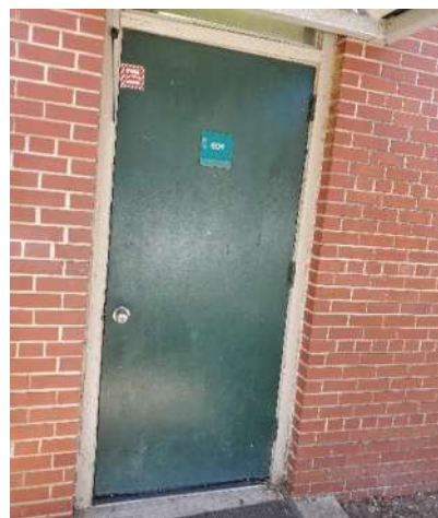
Photo #6 HA# F 14 – Fire Doors (multiple types)
