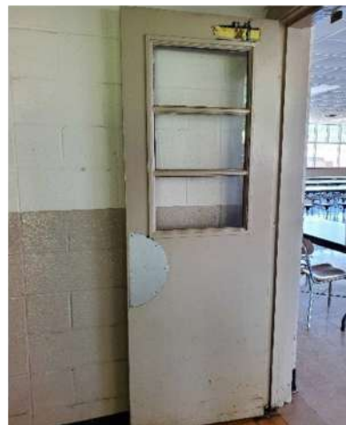
Photo #6 HA# E 25 – Fire Doors (multiple types)
