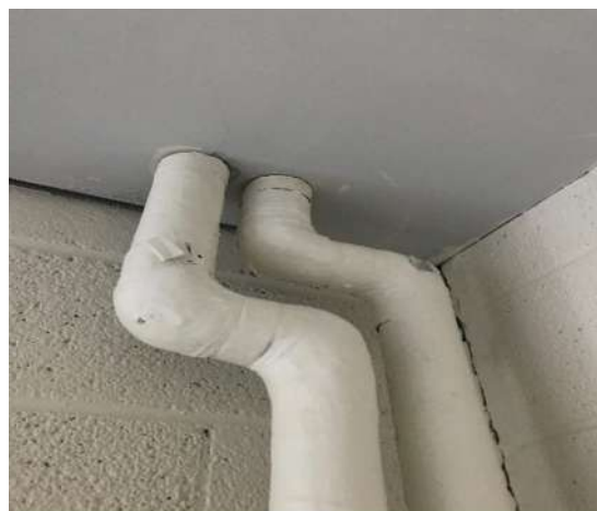
Photo #2 HA# B 3 – 1" Pipe Elbow Insulation
