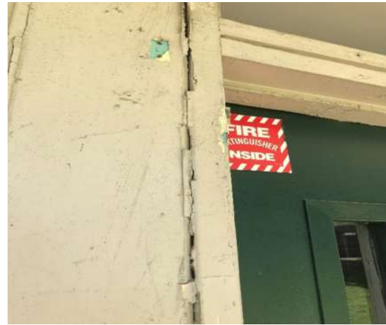
Photo #2 HA# C 6 – Exterior Door Caulk
