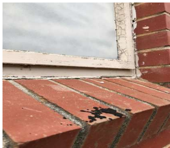
Photo #2 HA# F 8 – Exterior Window Frame Caulk
