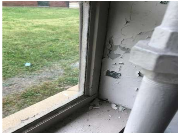
Photo #2 HA# A 6 – Interior Window Caulk
