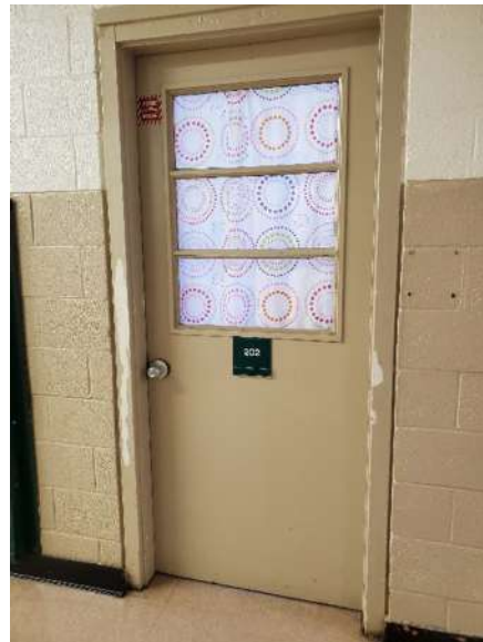
Photo #8 HA# A 26 – Fire Doors (multiple types)
