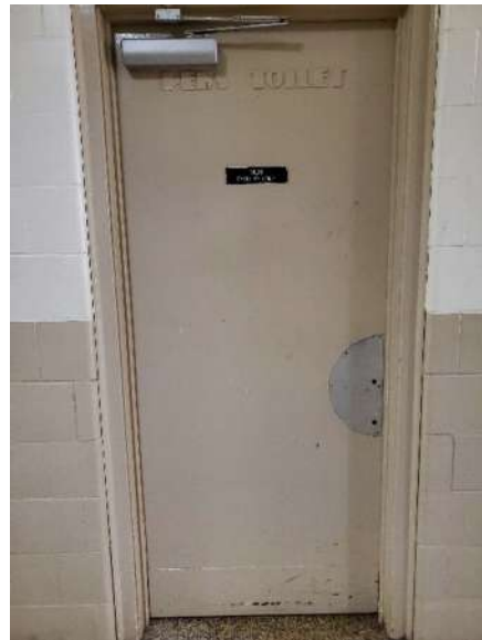
Photo #8 HA# B 26 – Fire Doors (multiple types)
