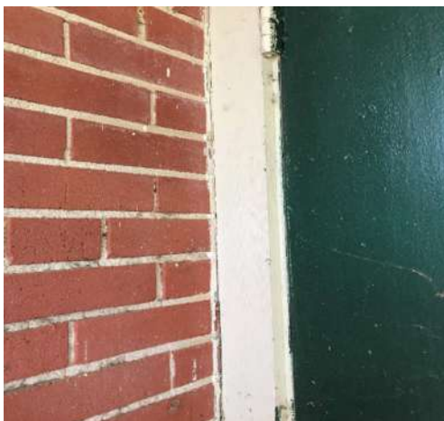
Photo #3 HA# F 9 – Exterior Door Caulk
