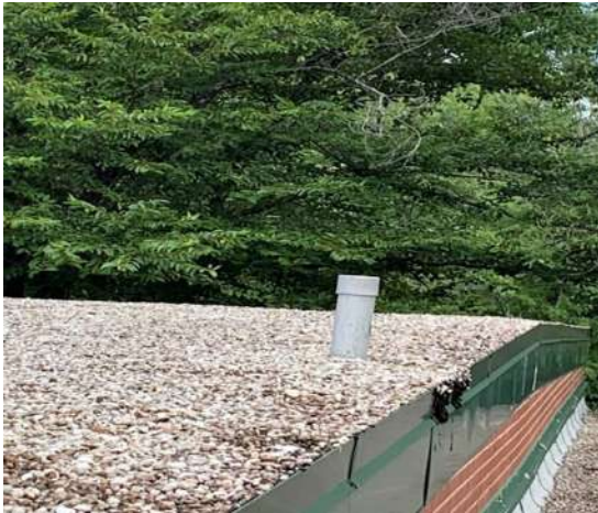
Photo #7 HA# FR 3 – Silver Paint Penetrations
