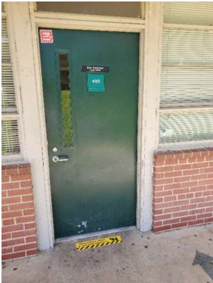
Photo #7 HA# D 12 – Fire Doors (multiple types)
