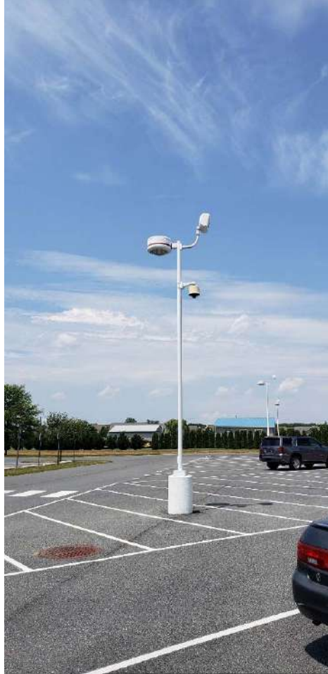
Photo #14 Typical Parking Lot Light Fixture
