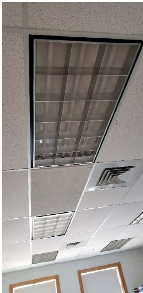
Photo #11 Typical Classroom Lighting Fixture
