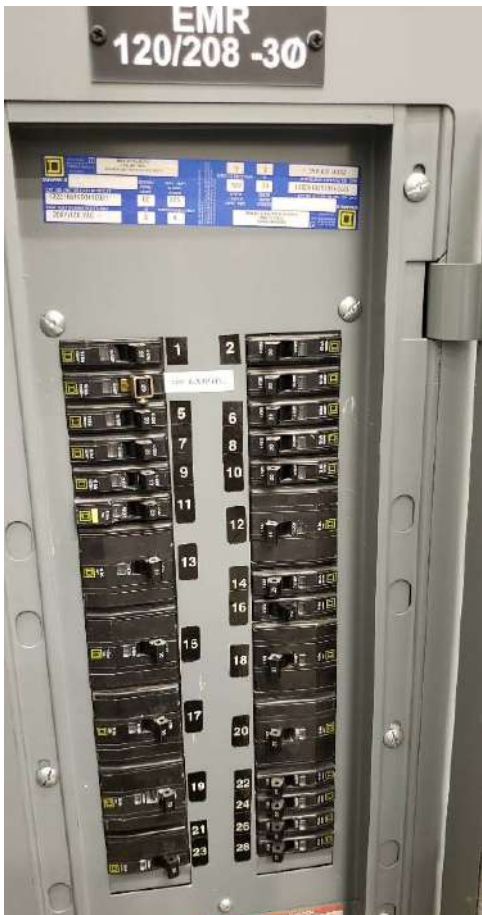
Photo #19 Typical Square D NQOD Branch Panelboard
