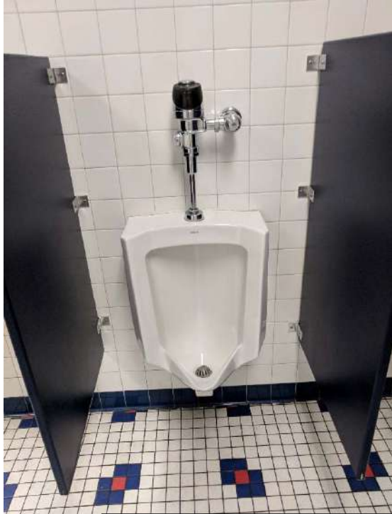
Photo #13 Typical Urinal
