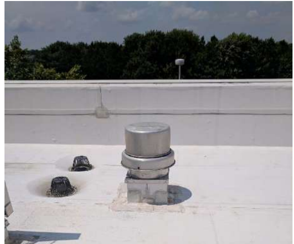
Photo #10 Typical Rooftop Exhaust Fan
