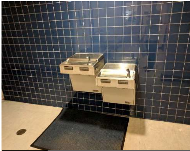
Photo #15 Typical Electric Water Coolers
