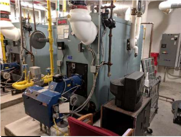
Photo #1 Boilers in Mechanical Room
