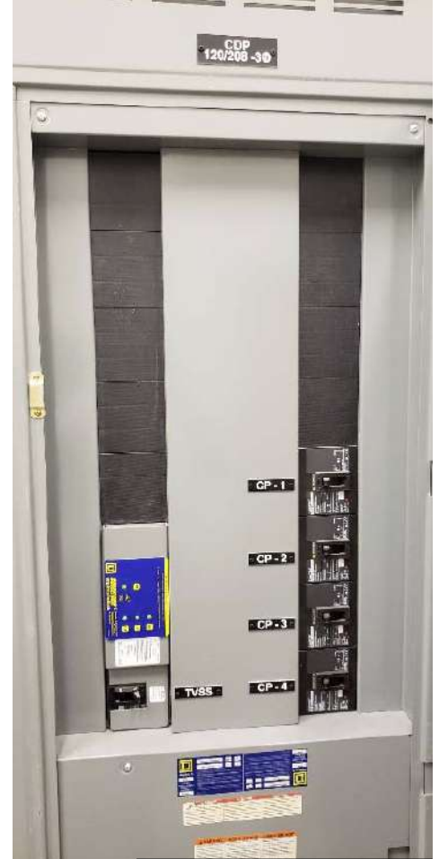
Photo #15 Typical Square D HCM Distribution Panelboard
