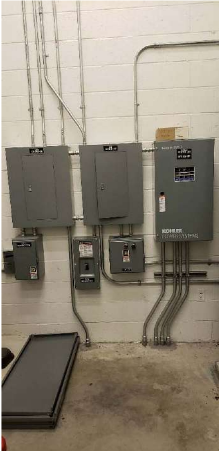
Photo #5 ATS-2 and Life Safety Panelboards
