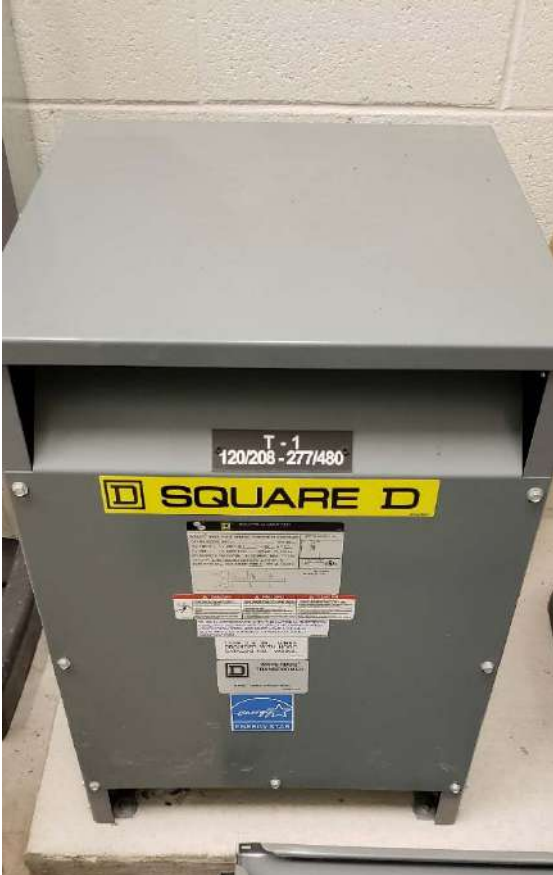
Photo #1 208V to 480V Boost Transformer
