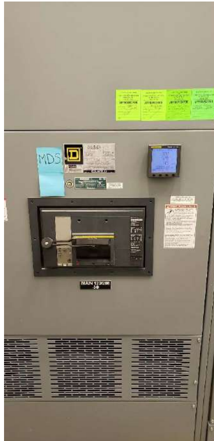
Photo #2 2500A Breaker in Main Switchboard
