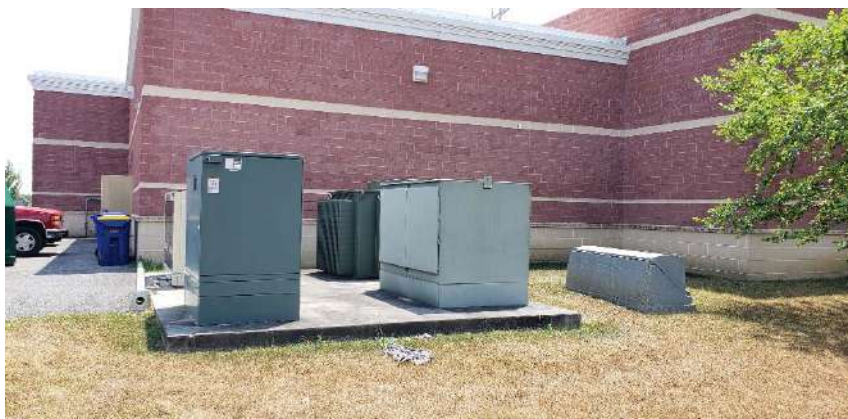
Photo #4 Exterior Electrical Equipment and Wallpack
