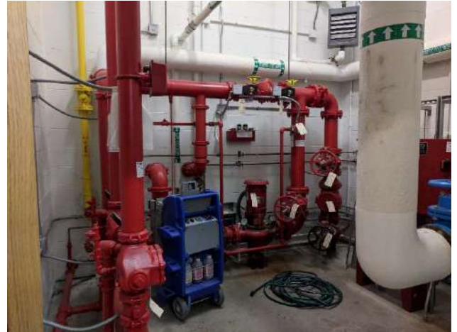
Photo #2 Domestic and Fire Protection Water Entrances
