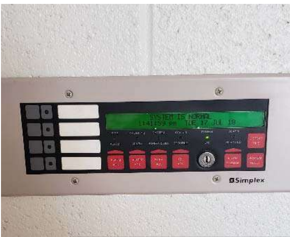
Photo #8 Fire Alarm Annunciator Panel
