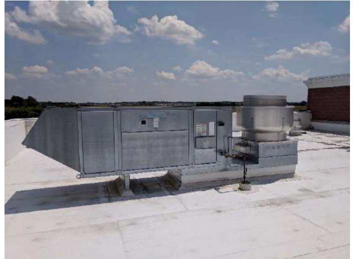
Photo #6 Kitchen Make Up Air Unit
