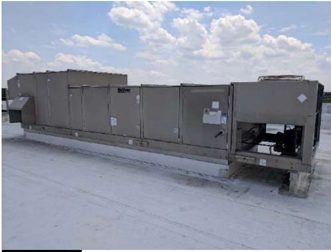
Photo #9 Typical Packaged RTU with Energy Recovery
