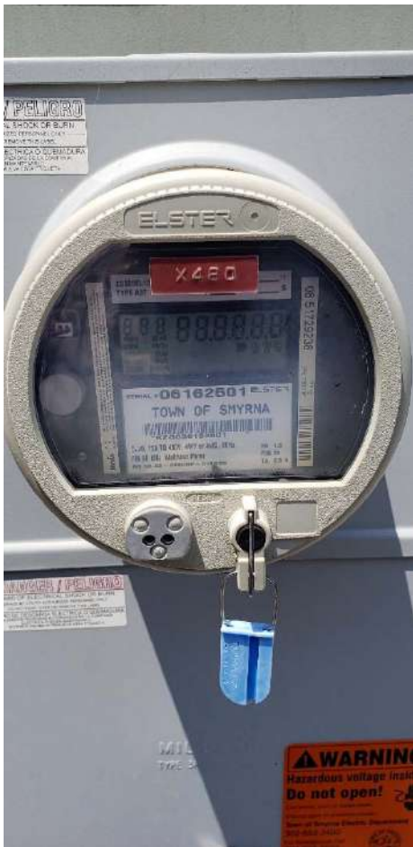
Photo #10 Primary Meter located on Metering Station
