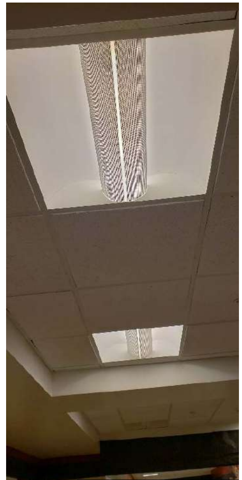
Photo #12 Typical Corridor Lighting Fixture
