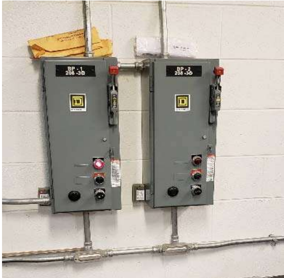
Photo #17 Typical Square D Motor Controllers
