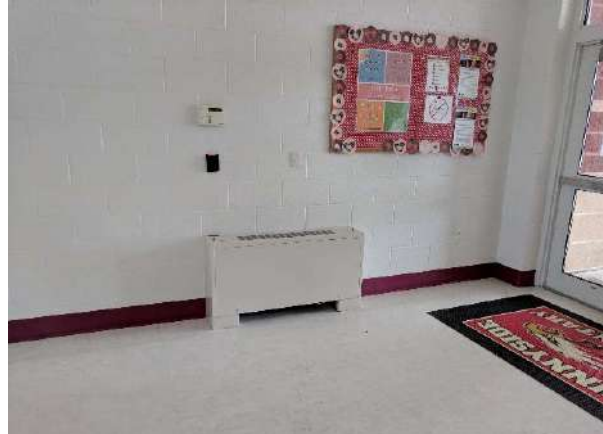
Photo #14 Typical Vestibule Cabinet Heater
