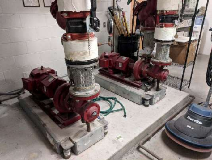
Photo #5 Heating Water Pumps in Mechanical Room
