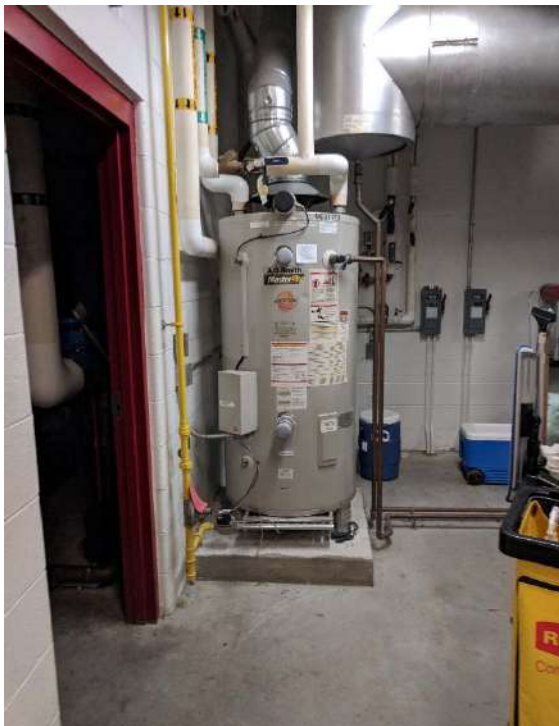
Photo #3 Domestic Water Heater
