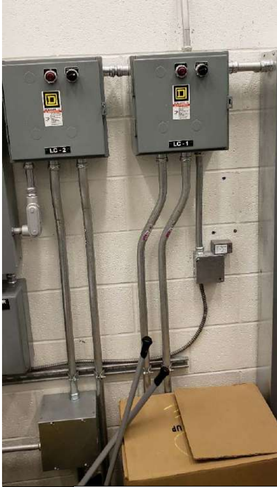
Photo #13 Typical Lighting Contactor for Site Lighting Fixtures
