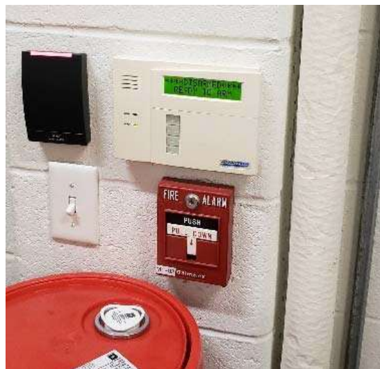
Photo #16 Typical Security Keypad and Card Reader
