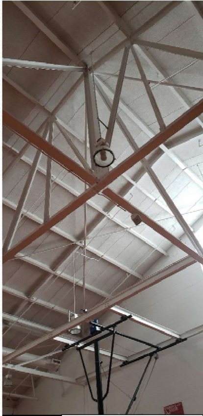
Photo #9 Gym Light Replaced with LED lamp
