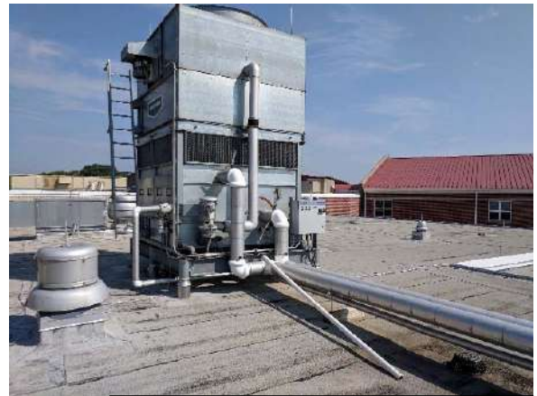
Photo #14 Abandoned Closed Circuit Cooler
