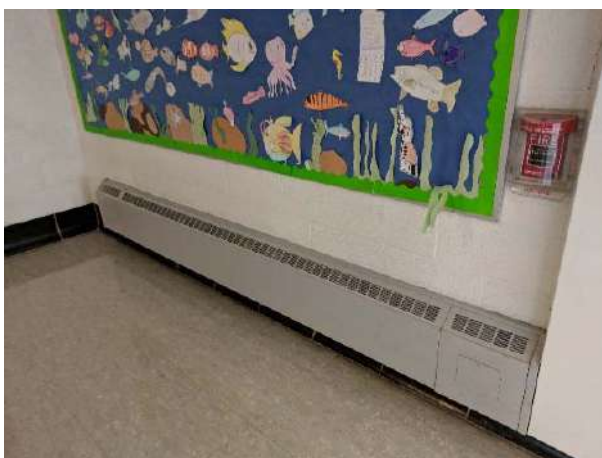
Photo #15 Typical Finned Tube Radiator
