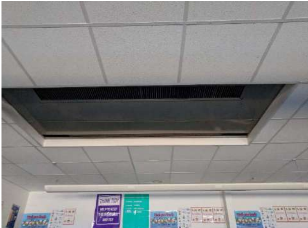
Photo #11 Typical Horizontal Unit Ventilator
