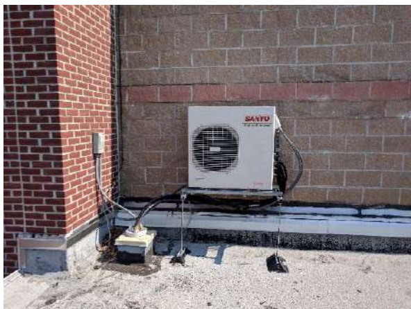
Photo #9 Typical Roof Mounted Condensing Unit
