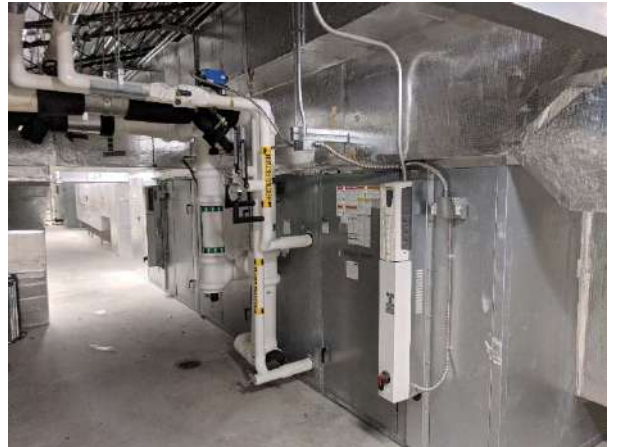
Photo #8 Typical Indoor AHU in Mechanical Mezzanine
