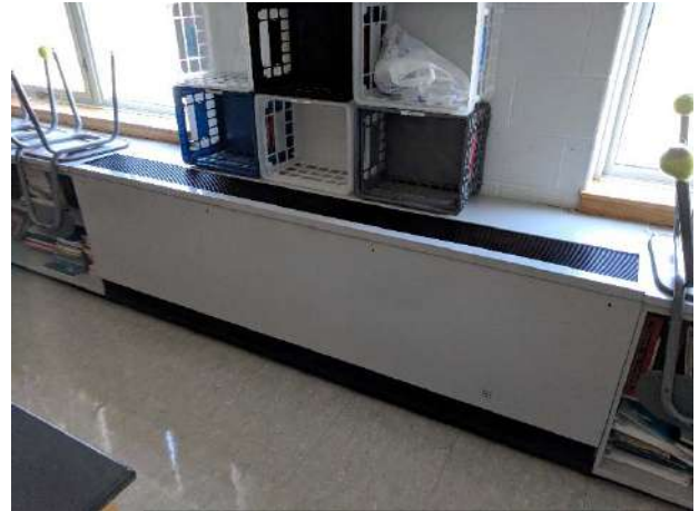
Photo #12 Typical Vertical Unit Ventilator
