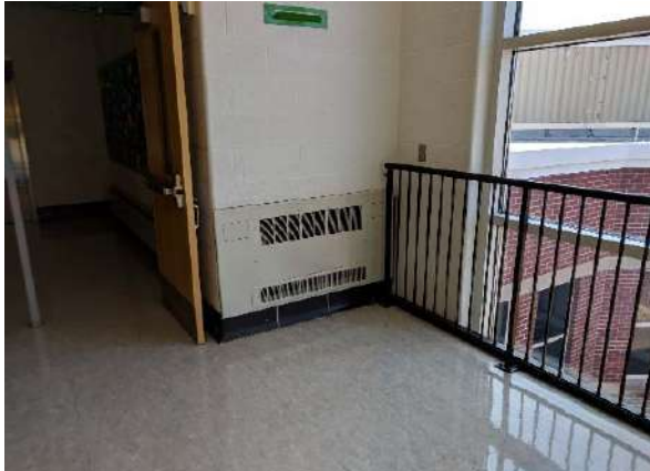
Photo #17 Typical Cabinet Heater
