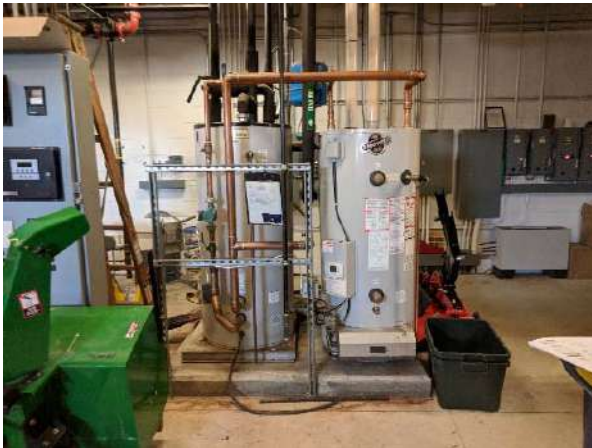
Photo #5 Domestic Hot Water Heaters
