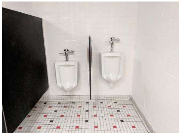
Photo #20 Typical Bathroom Urinals
