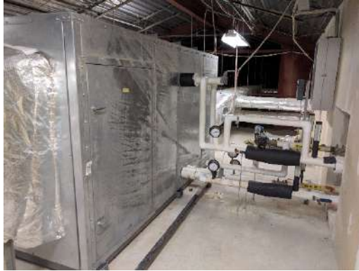
Photograph 2: ERU-2 in Mechanical Mezzanine
