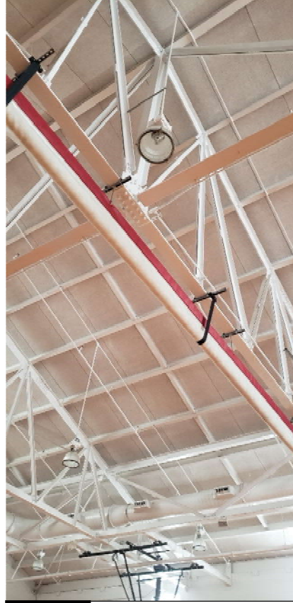
Photo #10 Gym Light with Metal Halide Lamp
