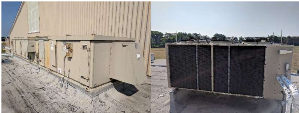
Photograph 3: Typical Rooftop Unit Split System
