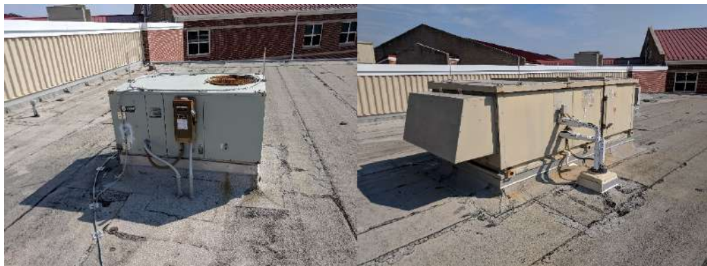
Photograph 4: Typical RTUs on Roof
