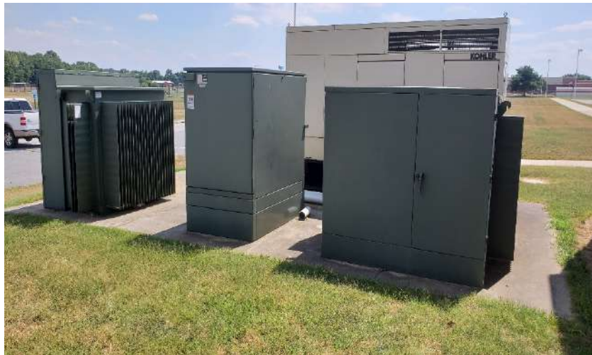
Photo #4 PHM-5 Switch, 208V and 480V Transformers, and 200kW Generator
