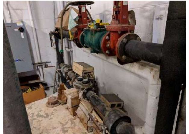
Photo #6 Domestic Water Entrance
