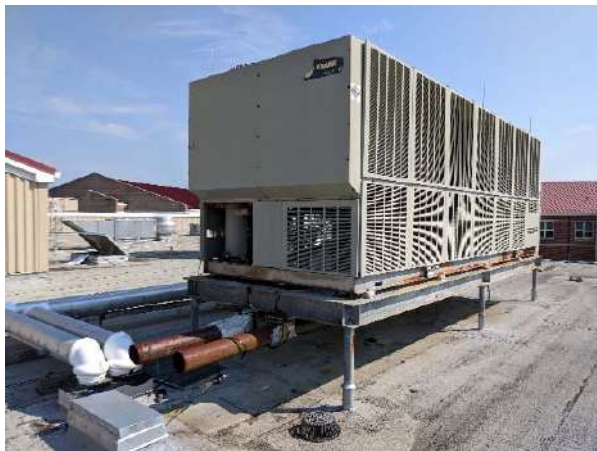
Photo #19 Abandoned Air Cooled Chiller
