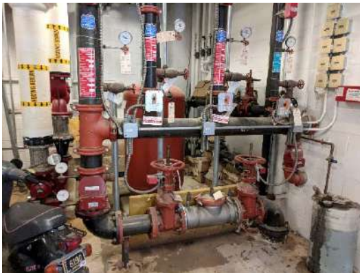
Photo #3 Fire Protection Zone Piping and Backflow Preventer
