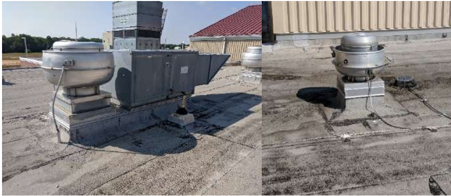
Photograph 5: Typical Make Up Air Unit and Dishwasher Exhaust Fan
