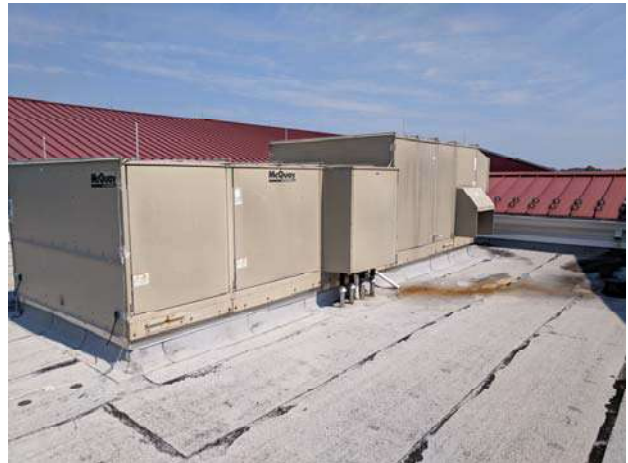
Photo #24 Typical Rooftop ERU
