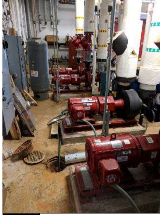
Photo #2 Secondary Heating and Cooling Pumps
