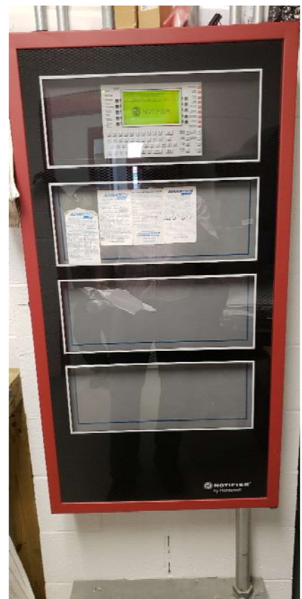
Photo #7 Fire Alarm Control Panel
