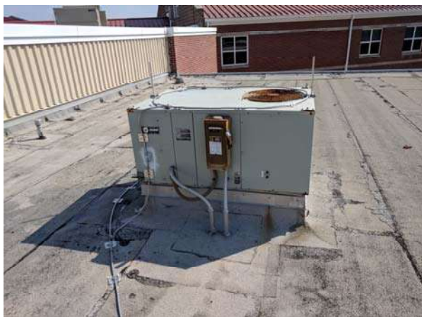
Photo #21 Typical RTU
