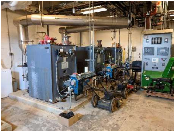
Photo #7 Abandoned Boilers
