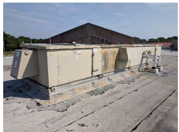
Photo #16 Typical 4-Pipe Rooftop Air Handling Unit
