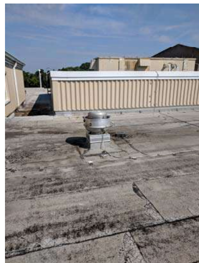
Photo #22 Typical Rooftop Exhaust Fan
