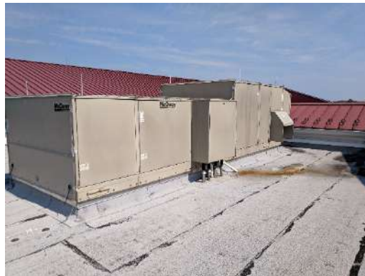
Photograph 1: ERU-5 on Roof
