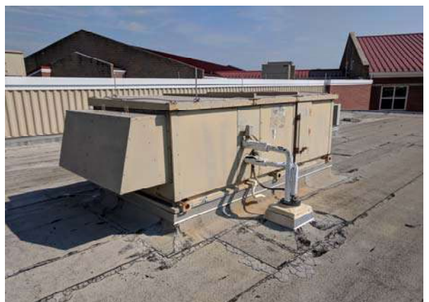
Photo #28 Typical 4-Pipe RTU
