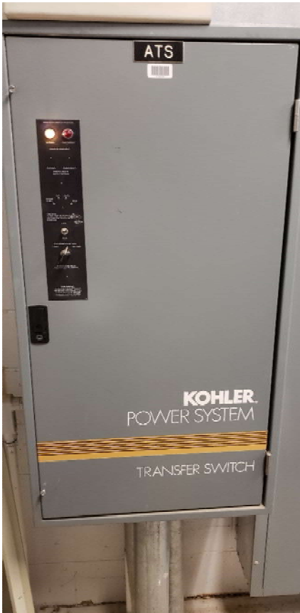
Photo #5 Automatic Transfer Switch
