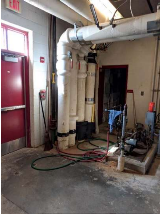
Photo #1 Primary Chilled and Heating Water Pipe Entrances
