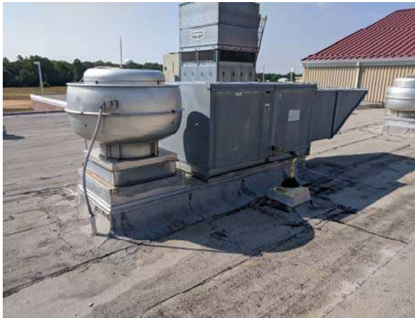
Photo #23 Typical Kitchen Ventilation Unit
