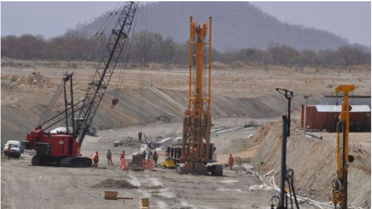
Part of the actual dam structure is already taking shape. The workers are busy at work on what looks like a huge floor of concrete.
