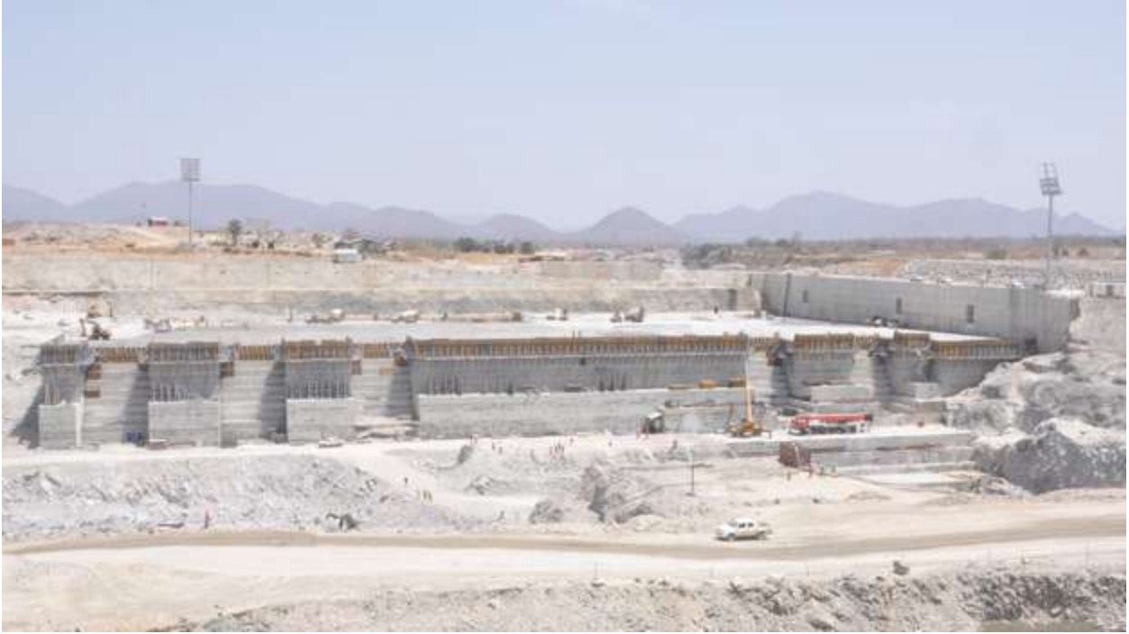
Some 8,500 people working at the site, where construction carries on 24 hours a day.
