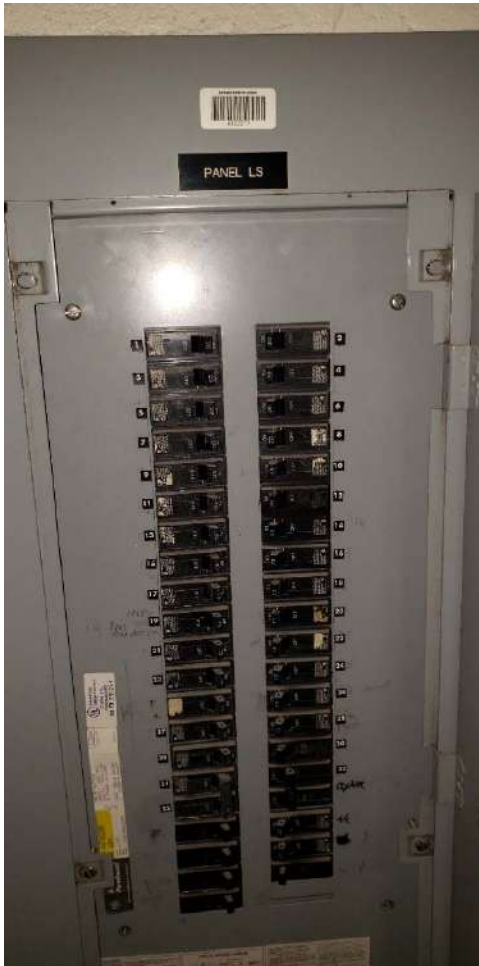
Photo #10 Typical Branch Panelboard installed in 1993
