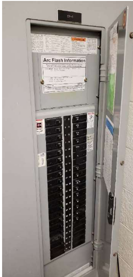
Photo #11 Typical Branch Panelboard installed in 2002
