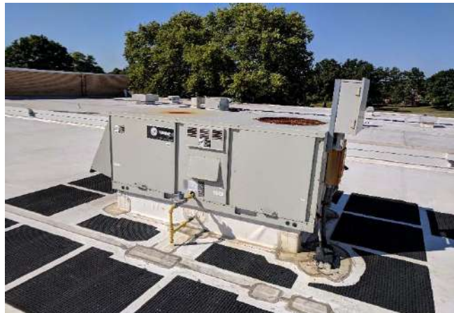
Photo #8 RTU Serving Library
