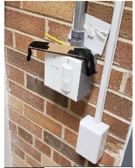
Photo #20 Typical Wall Mounted Occupancy
