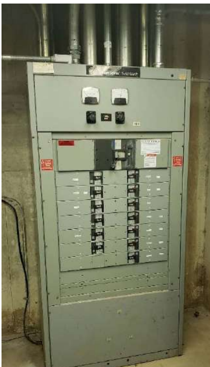
Photo #7 Switchboard MDP
