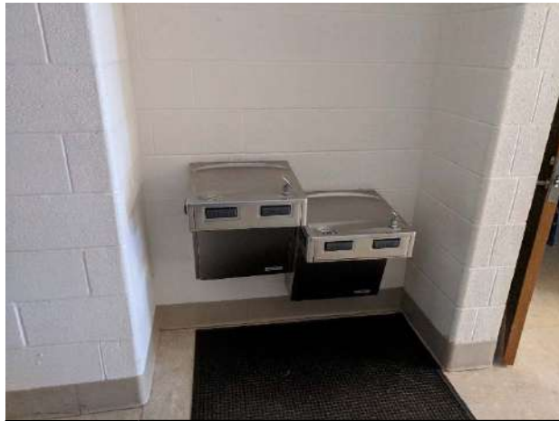
Photo #21 Typical Water Fountain
