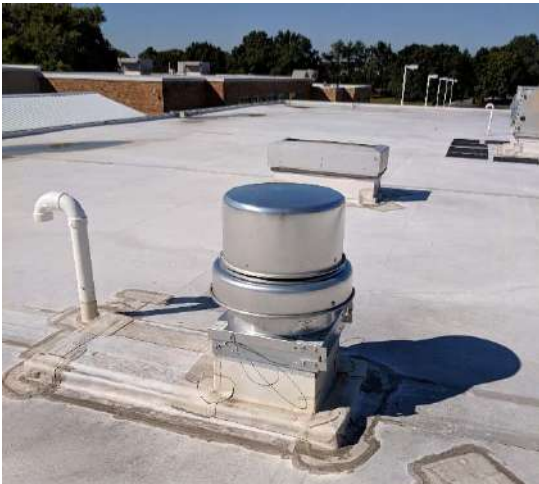
Photo #17 Typical Exhaust Fan
