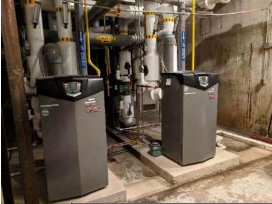
Photo #15 Typical Boilers in Mechanical Room
