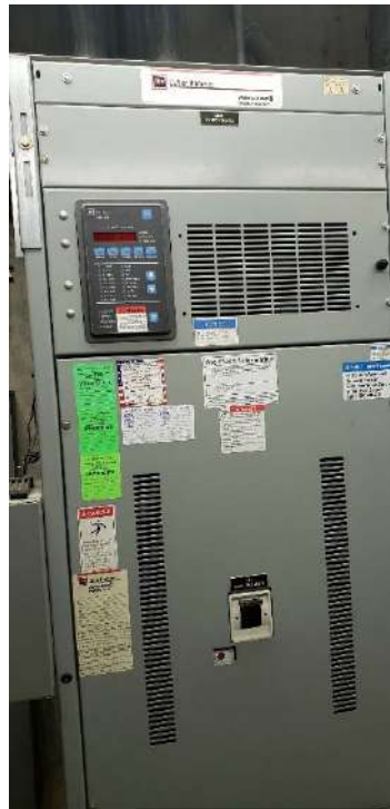
Photo #8 Switchboard MDS
