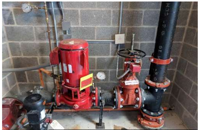
Photo #6 Fire Pump
