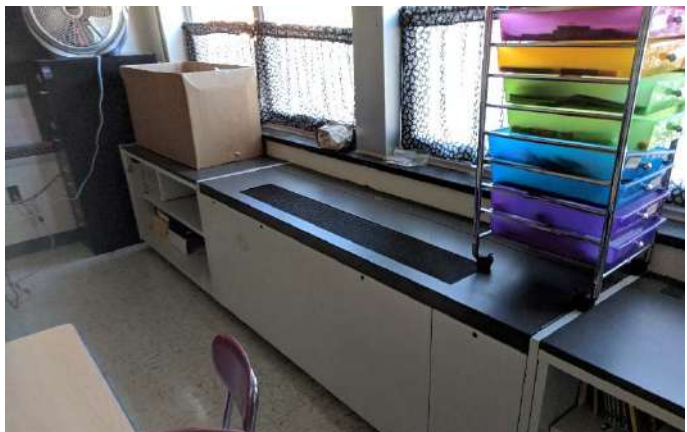
Photo #10 Typical Unit Ventilator
