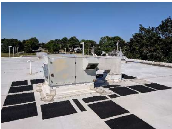
Photo #9 Typical Energy Recovery Unit
