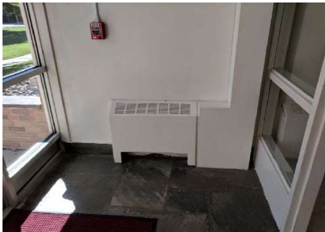
Photo #23 Typical Vestibule Cabinet Heater
