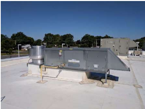
Photo #7 Kitchen Makeup Air and Exhaust Unit
