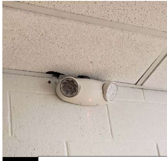
Photo #19 Typical Wall Mounted Emergency Light
