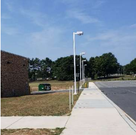
Photo #16 Typical LED Parking Lot Lights
