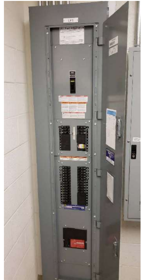
Photo #12 Typical Branch Panelboard installed in 2015
