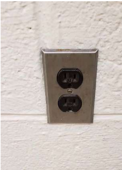
Photo #18 Typical Receptacle
