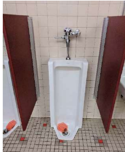
Photo #22 Typical Urinal
