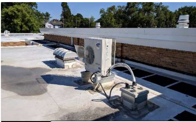
Photo #20 Typical Split DX Condenser Unit
