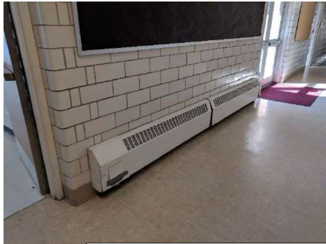
Photo #18 Typical Fin Tube Radiator
