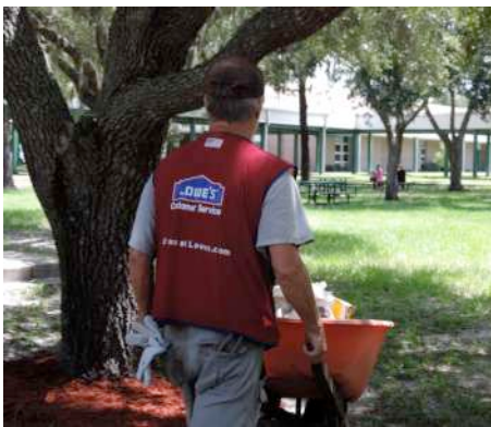
A Lowe's Hero helps to construct the outdoor classroom for our campus.
