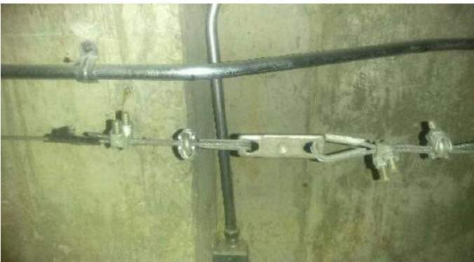
FIRE CURTAIN: IMPROPER TERMINATIONS
