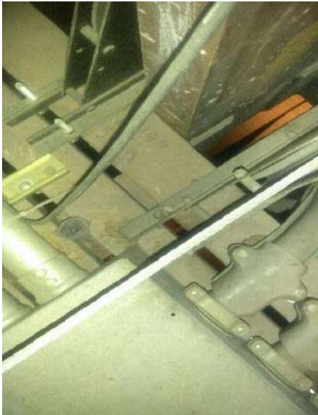
MISSING/LOOSE J-BOLTS & U-BRACKETS
