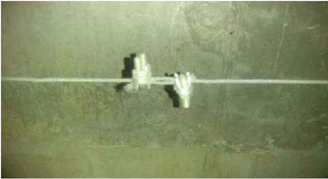
FIRE CURTAIN: IMPROPER TERMINATIONS
