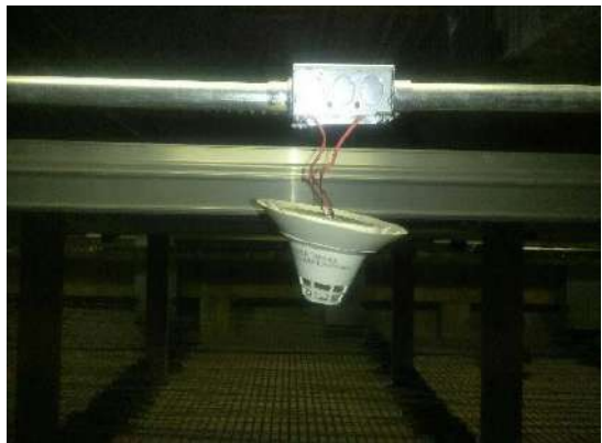
BROKEN FIRE SENSORS
