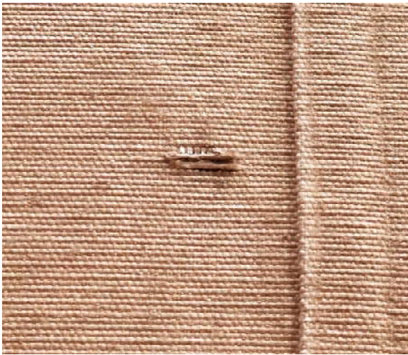
RIP IN FIRE CURTAIN
