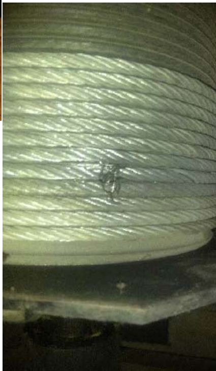
DAMAGED CABLE ON CLANCY MOTOR 1,
