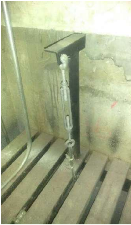
TURNBUCKLES FOR FIRE CURTAIN NOT MOUSED
