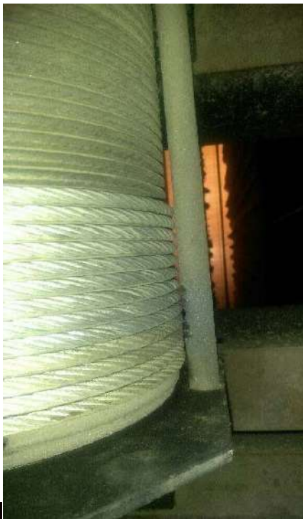
RUBBING CABLES ON DRUMSHAFTS
