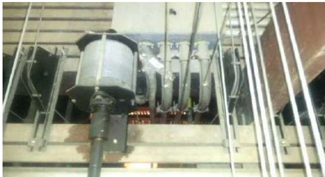
BROKEN CABLE PROTECTOR
