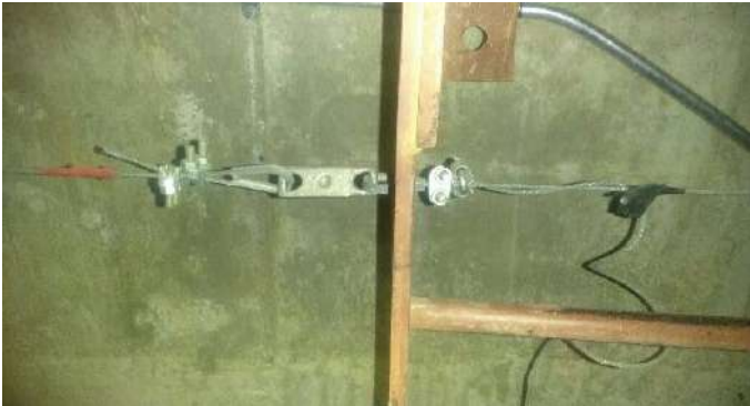
FIRE CURTAIN: IMPROPER TERMINATIONS
