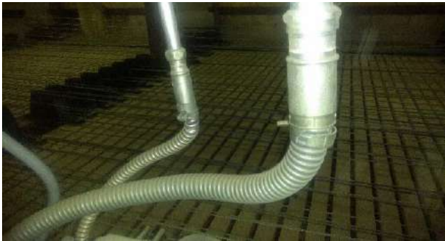
BROKEN CABLE CONNECTORS
