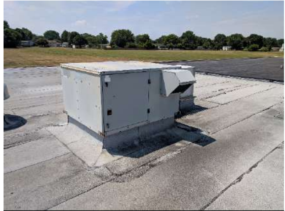
Photograph #5 – Typical Energy Recovery Unit
