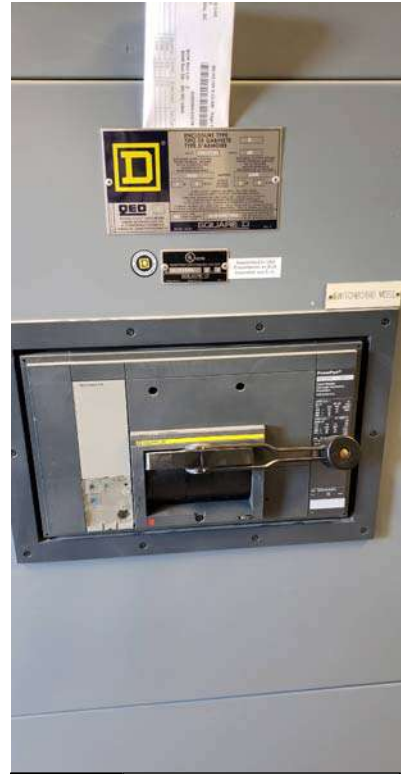
Photo #9 Switchboard MDS2
