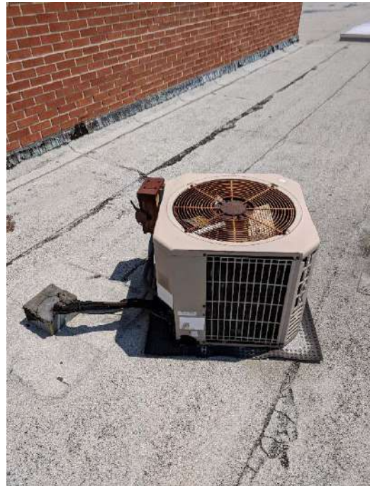
Photo #8 DX Split System Condensing Unit
