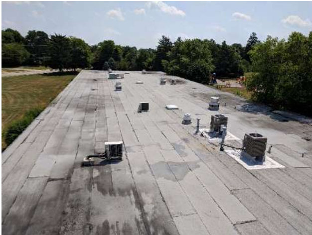
Photo #3 D Wing Roof Mechanical Equipment
