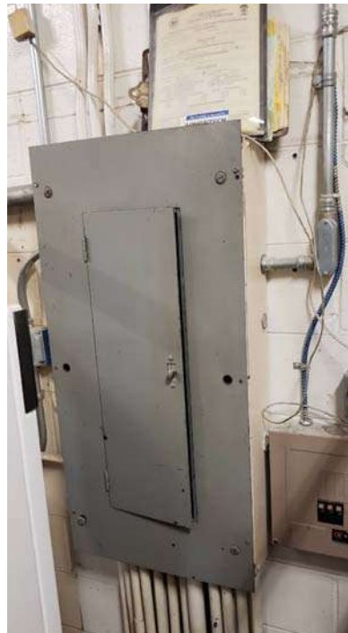
Photo #5 Panelboard E
