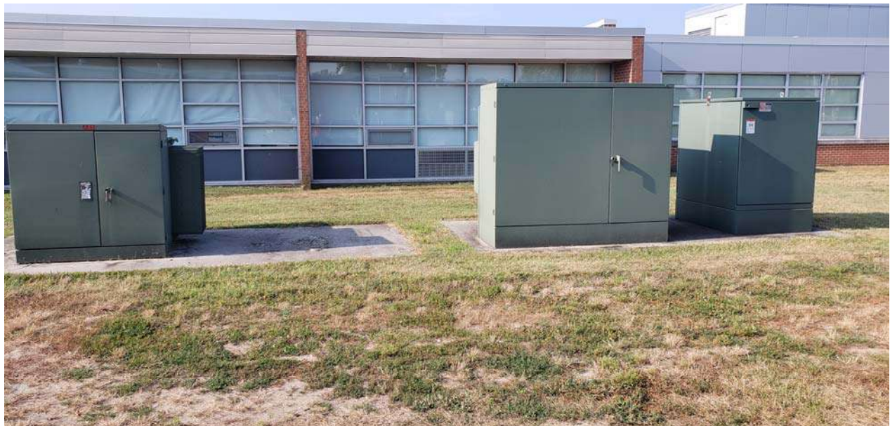
Photo #10 Transformer and PMH-3 Switch
