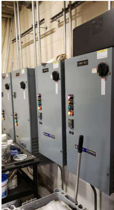
Photo #20 Typical VFD
