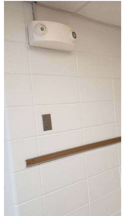
Photo #21 Typical Wall Mounted Emergency Light Fixture
