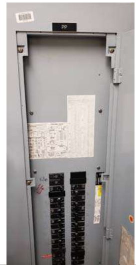
Photo #18 Typical Panelboard installed in 1993
