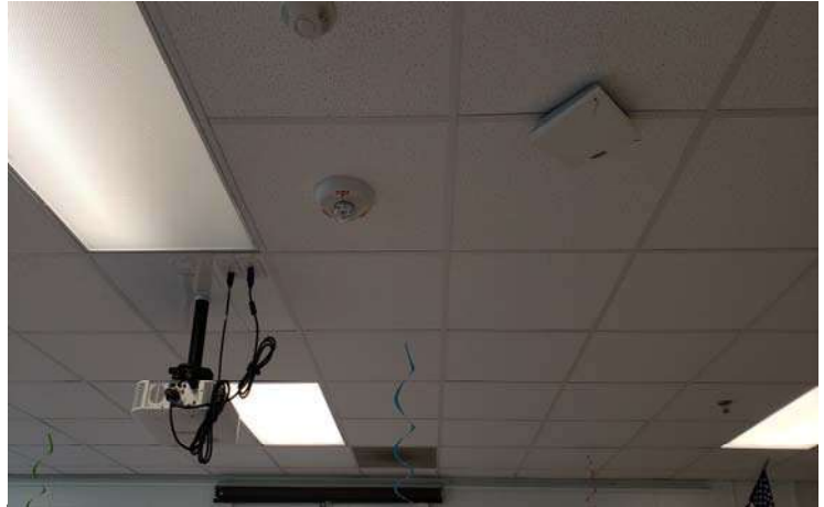
Photo #12 Typical Classroom with Occupancy Sensor
