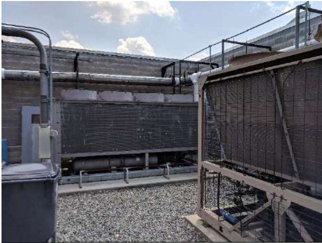
Photo #1 Air Cooled Chillers
