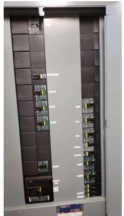
Photo #6 Panelboard MDP
