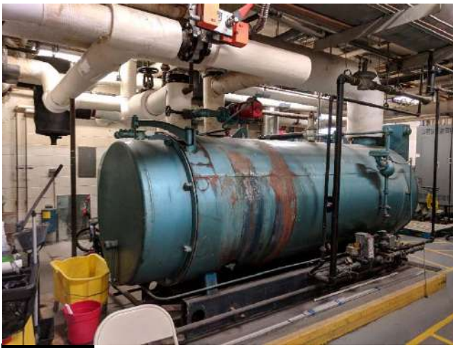
Photo #9 Backup Boiler in Mechanical Room
