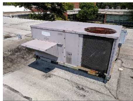
Photograph #4 – RTU Serving Library
