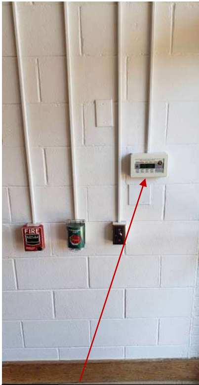
Photo #1 Fire Alarm Annunciator Panel
