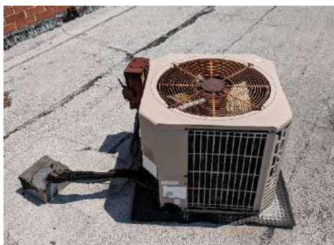
Photograph #3 – DX Split System Condensing Unit
