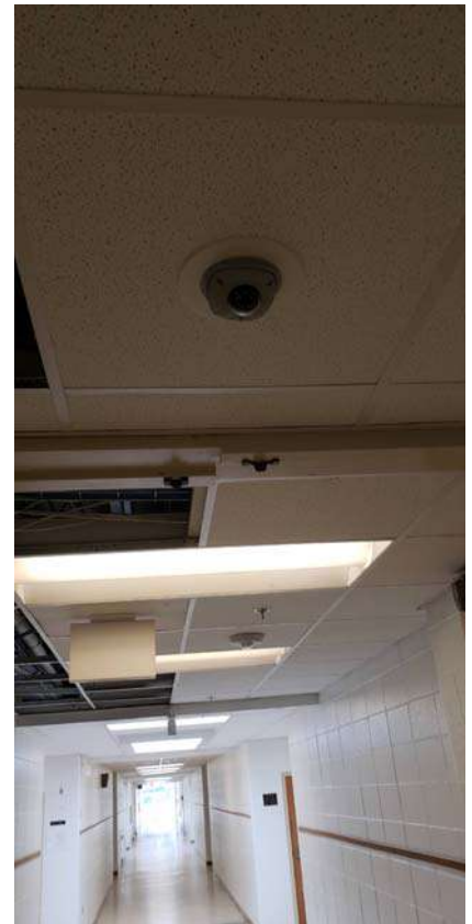
Photo #15 Typical Interior Video Surveillance
