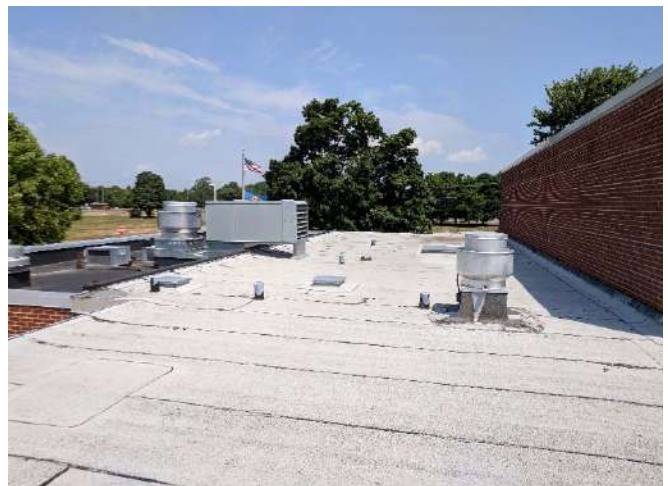
Photo #6 Kitchen Mechanical Equipment on Roof
