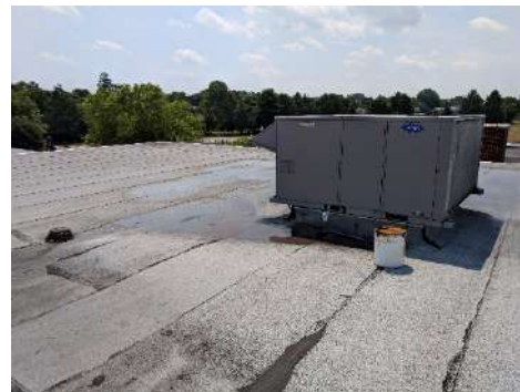
Photograph #2 – Cafeteria RTU
