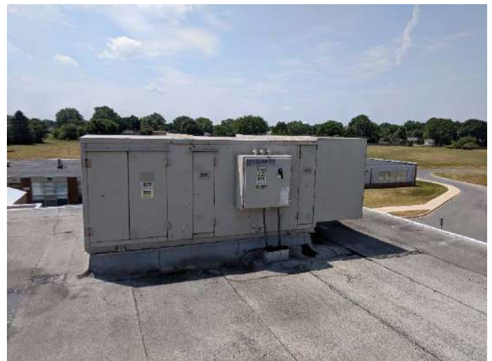
Photo #10 Gym RTU
