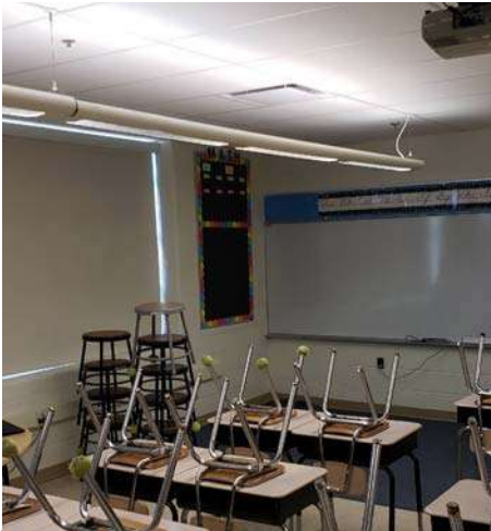
Photo #11 Typical 2006 Addition Classroom Lighting
