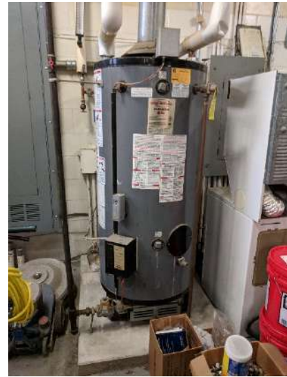
Photograph #6 – Domestic Water Heater
