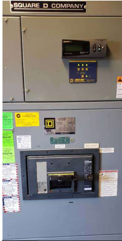
Photo #8 Switchboard MDS1
