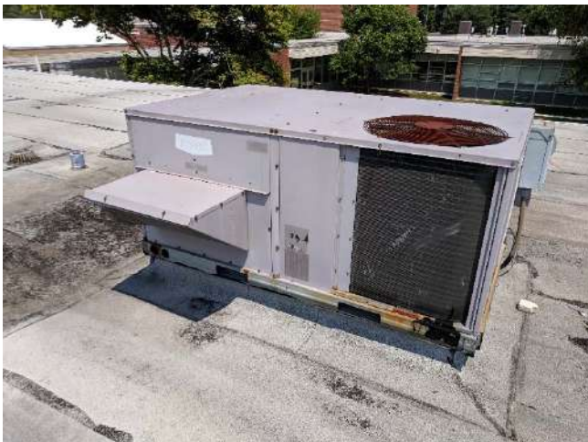
Photo #11 RTU serving Library
