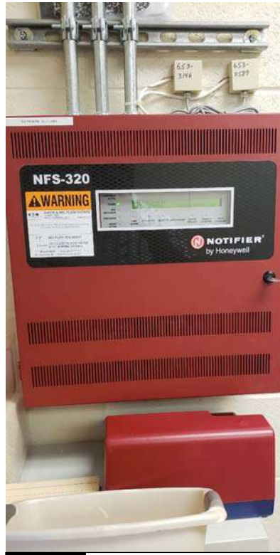
Photo #2 Fire Alarm Control Panel
