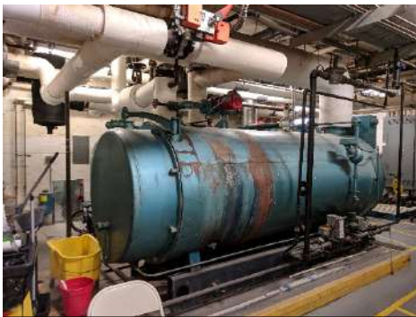
Photograph #1 – Backup Boiler in Mechanical Room
