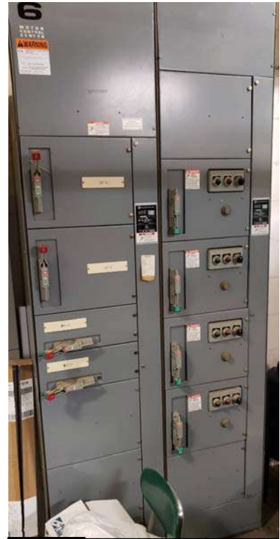
Photo #3 Motor Control Center
