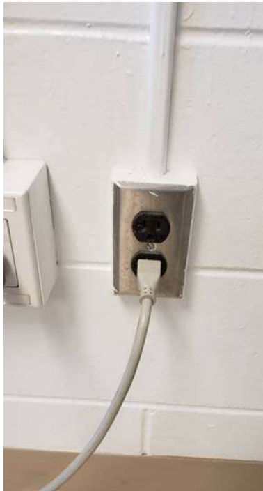
Photo #19 Typical Surface Mounted Receptacle
