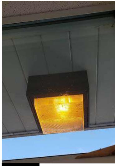
Photo #17 Typical Light under Canopy
