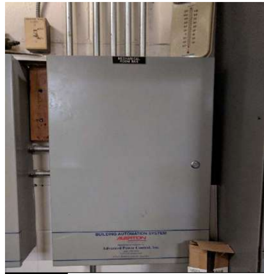
Photo #2 BAS Control Panel
