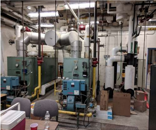
Photo # 12 Boilers in Mechanical Room
