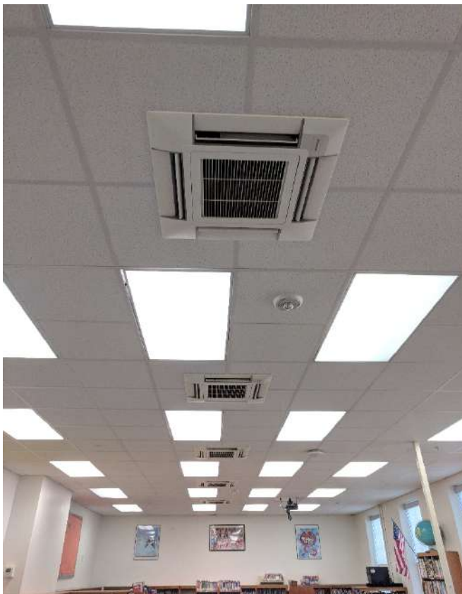
Photo #3 Ceiling Cassettes-Library
