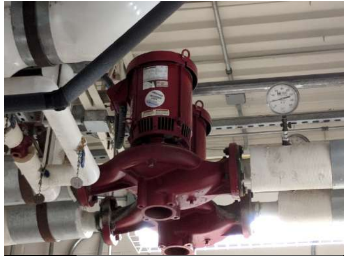
Photo #9 Heating Hot Water Pumps in Mechanical Room
