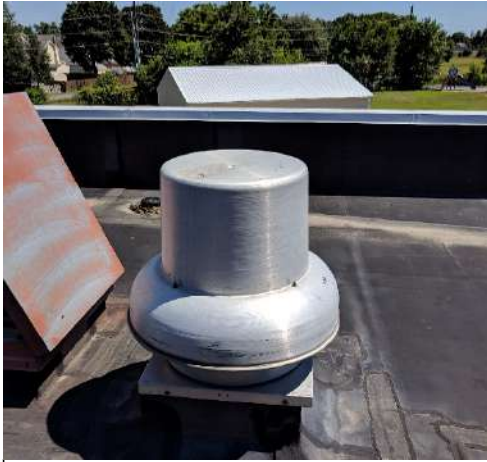
Photograph #3 – Typical Exhaust Fan
