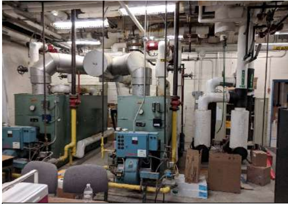
Photograph #1 – Boilers in Mechanical Room
