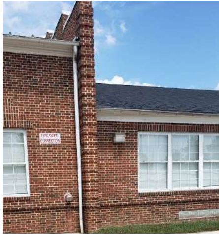
Photo #13 Typical Exterior Wall Pack
