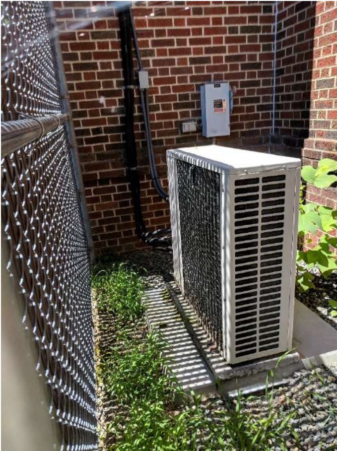
Photo #8 Ground Mounted Split DX Condensing Unit
