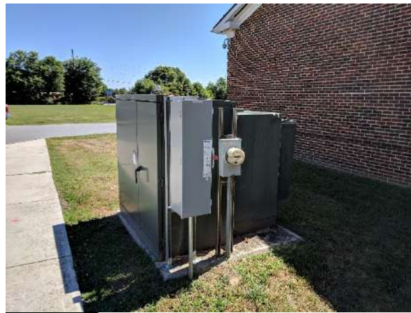
Photo #16 Transformer, Meter, and Disconnect for Fire Pump
