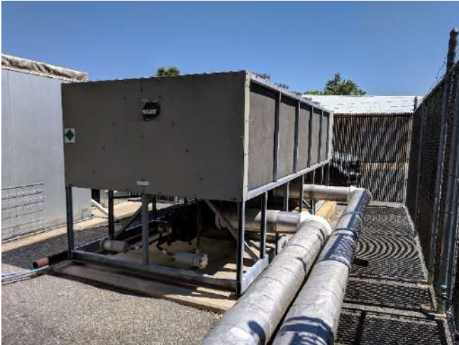
Photo #1 Air Cooled Chiller in Mechanical Yard
