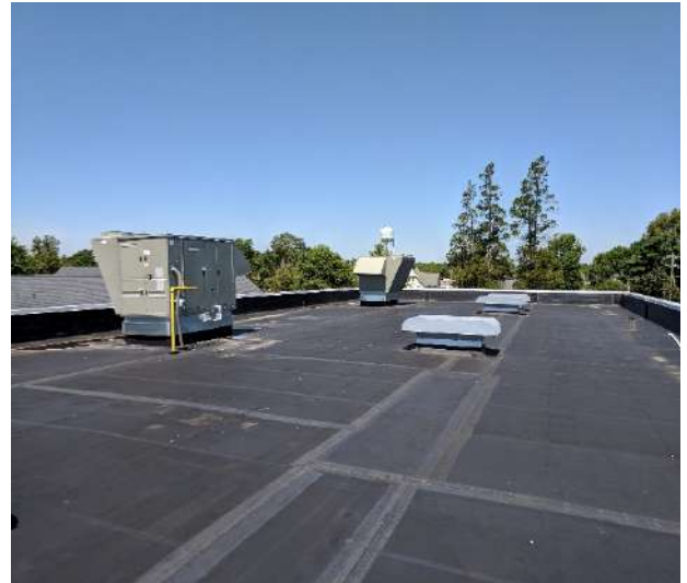
Photo #13 RTUs serving Cafeteria, Gym, and Auditorium
