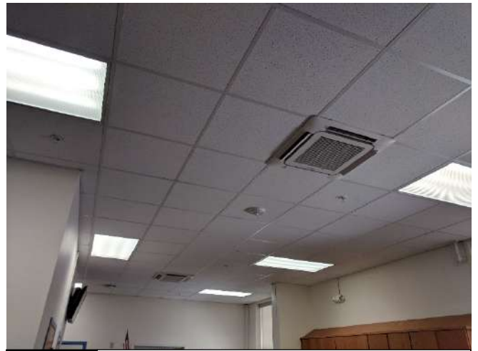
Photo #2 Ceiling Cassettes-Front Office
