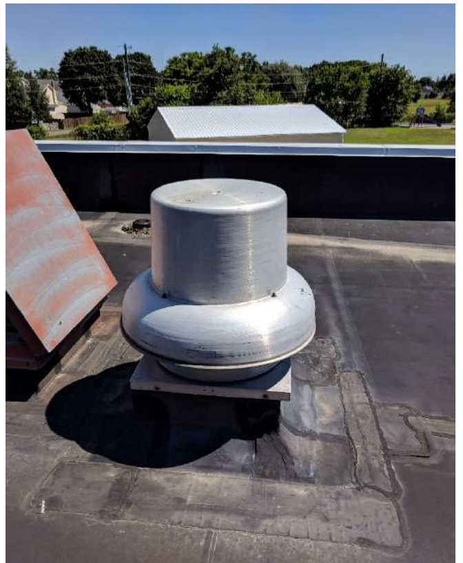
Photo #11 Typical Roof Mounted Exhaust Fan
