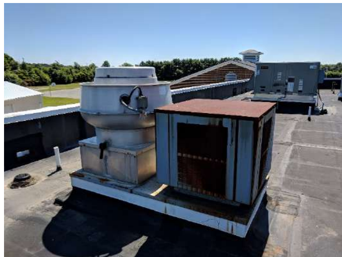
Photo #10 Kitchen Ventilation System
