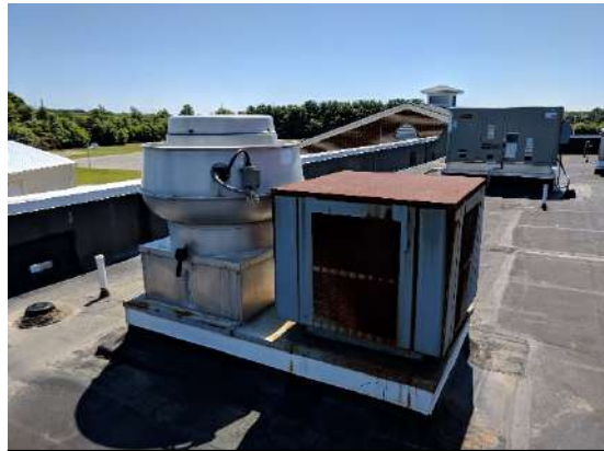
Photograph #2 – Kitchen Ventilation Unit
