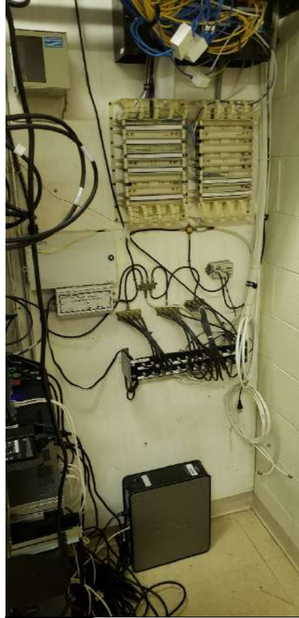
Photo #2 Telephone CATV incoming service
