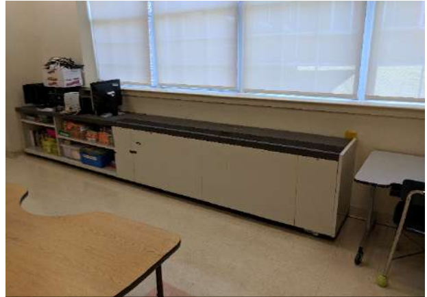
Photograph #4 – Typical Classroom Unit Ventilator
