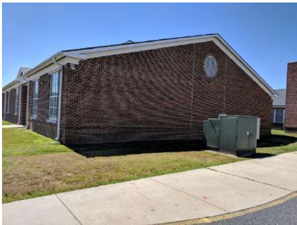
Photo #15 Exterior Lighting on the 2006 Addition
