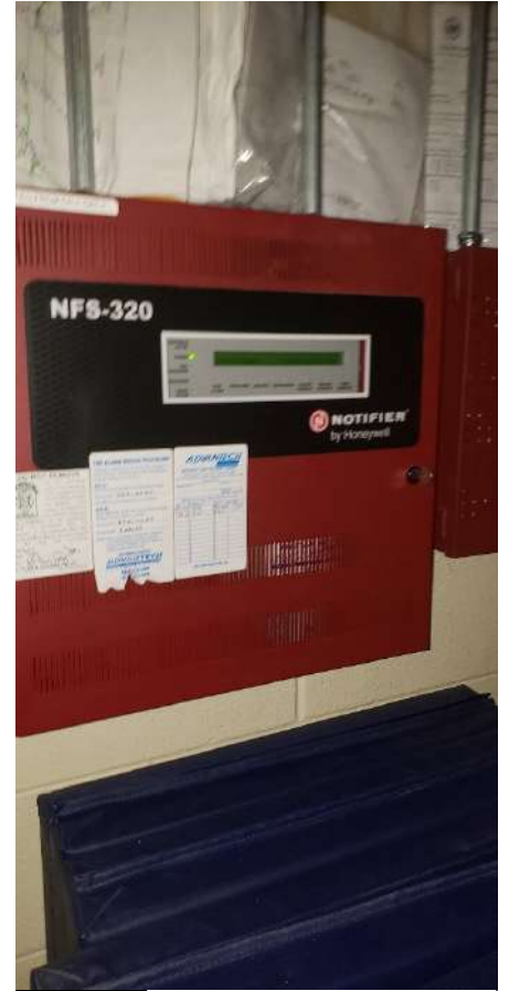
Photo #3 Fire Alarm Control Panel
