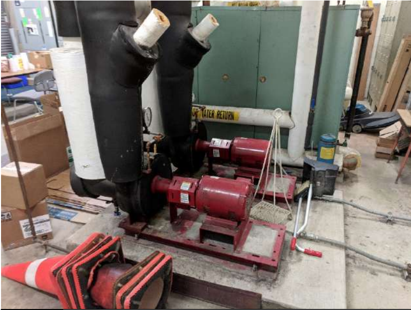
Photo #5 Chilled water Pumps in Mechanical Room
