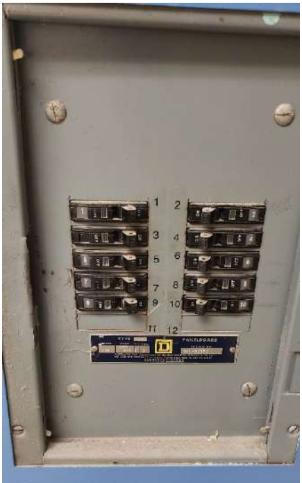
Photo #4 Panelboard LPB
