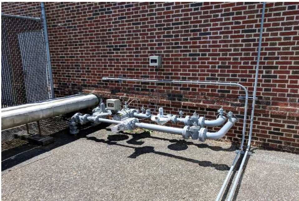
Photo #7 Gas Meter
