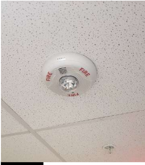
Photo #7 Typical Ceiling Mounted Fire Alarm Device
