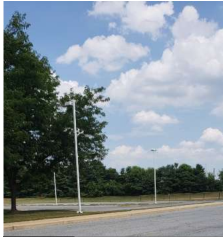
Photo #14 Typical Parking Lot Pole Lights
