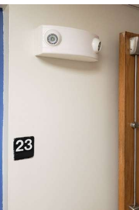
Photo #6 Typical Wall Mounted Emergency Light
