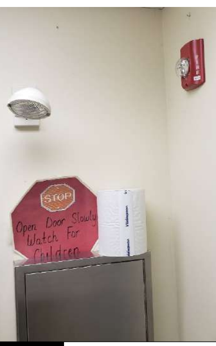
Photo #5 Wall Mounted FA device in typical Bathroom
