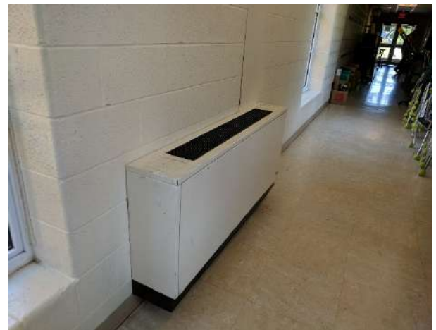
Photo #15 Typical Fan Coil Unit
