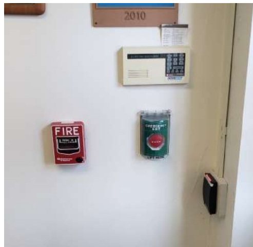
Photo #11 Fire Alarm Pull Station, Card Reader, and Security Keypad
