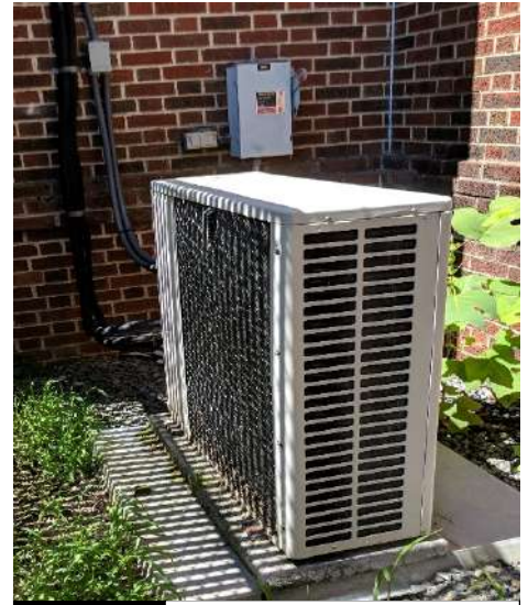
Photo #9 Exterior Disconnect on Wall
