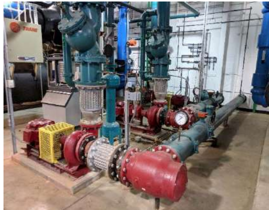
Photo #2 Condenser pumps
