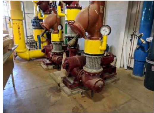
Photo #7 Primary Heating Water Pumps
