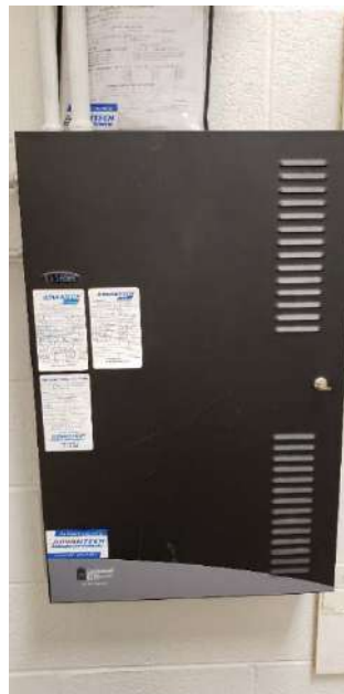
Photo #10 Fire Alarm Control Panel
