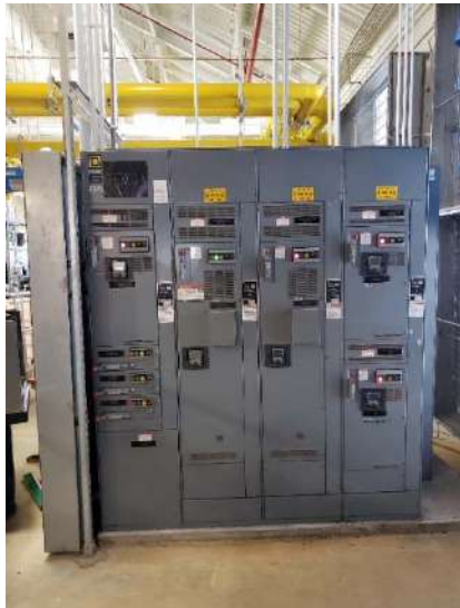
Photo #2 Typical Motor Control Center (MCC)
