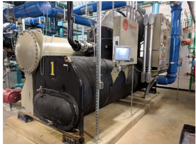
Photo #9 Typical Chiller
