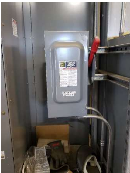
Photo #4 Typical Disconnect Switch
