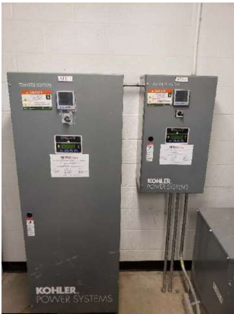
Photo #9 Automatic Transfer Switches
