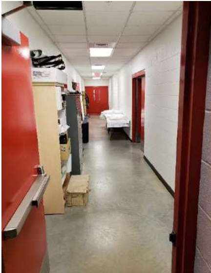
Photo #1 Typical Recessed Fluorescent 2'x4' Light Fixtures
