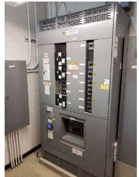
Photo #6 Main Switchboard CPMPP
