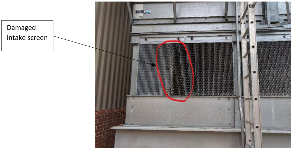
Photograph 1: Cooling Tower Damage
