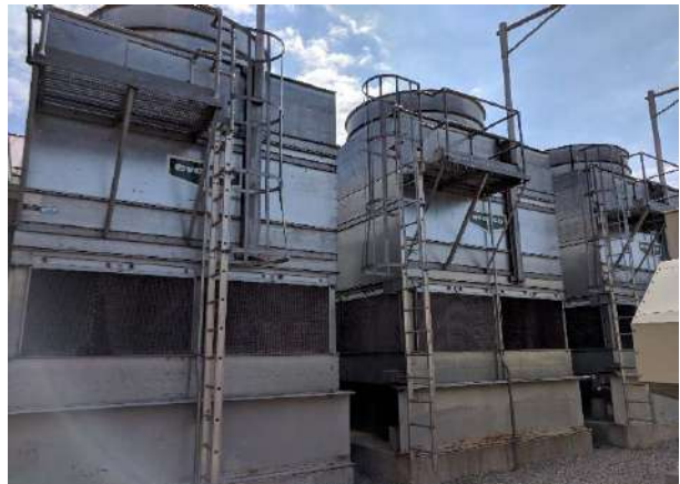
Photo #4 Cooling Towers
