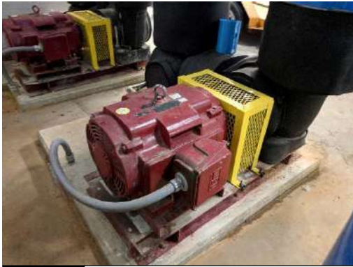
Photo #6 Primary Chilled Water Pumps
