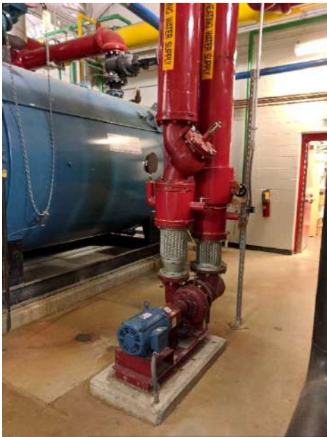
Photo #8 Typical Boiler Pump
