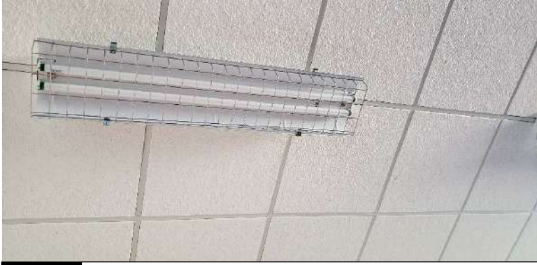
Photo #7 Typical Surface Mounted Fluorescent Strip Light
