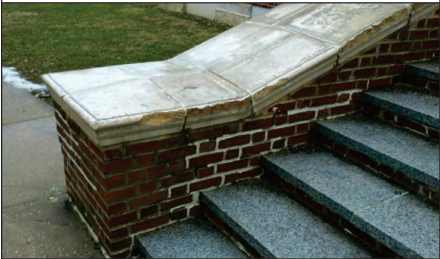
JBM Monumental stair – wall deterioration do to age
