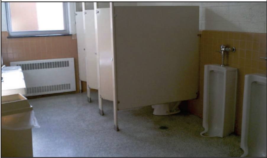
SES Aging public restrooms – need modern updates & ADA installation
