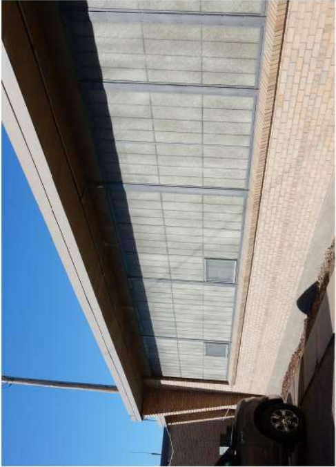
The current high school windows do not allow adequate light and are not weatherproof.
