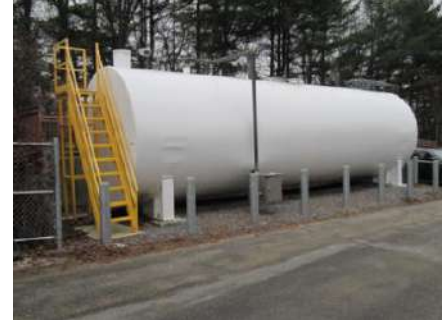
20,000 gallon oil tank located at NHS
