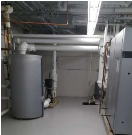
New gas fired burners at NMS
