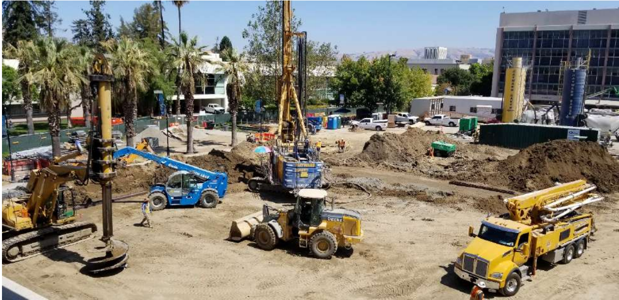
Photo: Predrill, Soil Mixing Equipment, loader, Forklift, Silos and on-site batching. Concrete pump truck on the right – for foundation work, not related DSM
