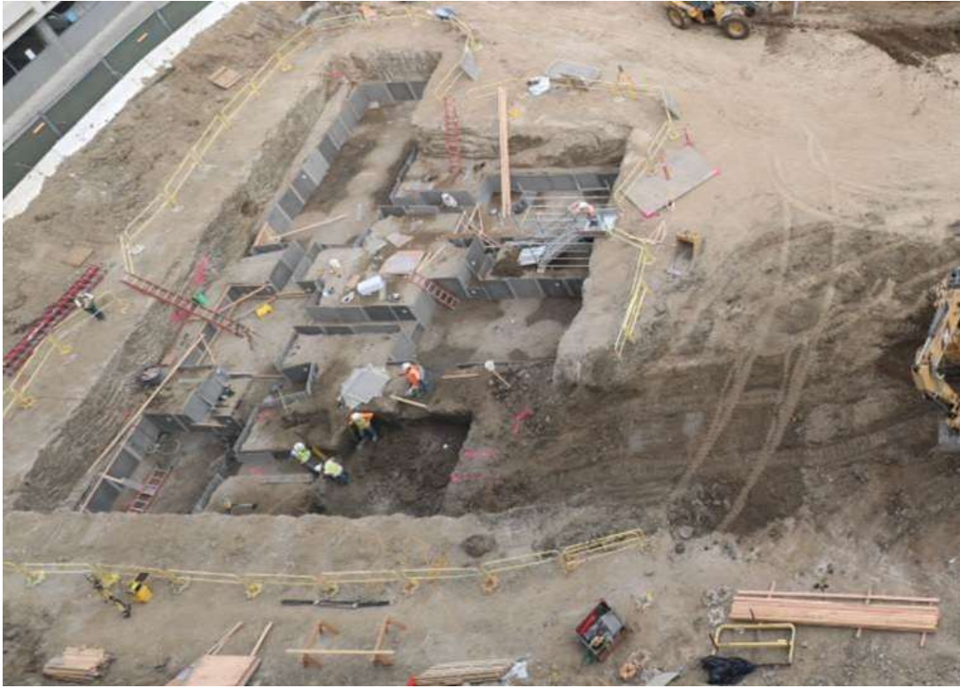
Photo: Visual representation of interlocking cellular grid soil mixed column shown after excavation.
