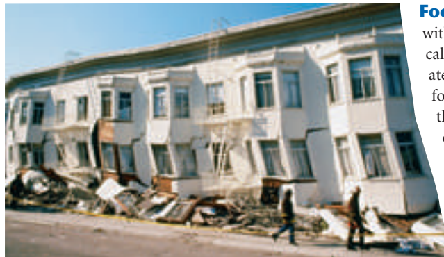
Figure 1 This damage occurred in San Francisco’s Marina District from the 1989 Loma Prieta earthquake.
