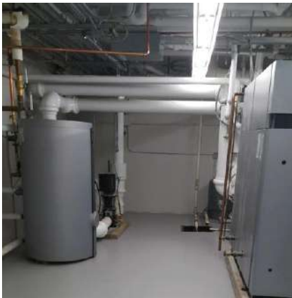
New gas fired burners at NMS
