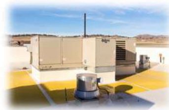
HVAC and ductwork
