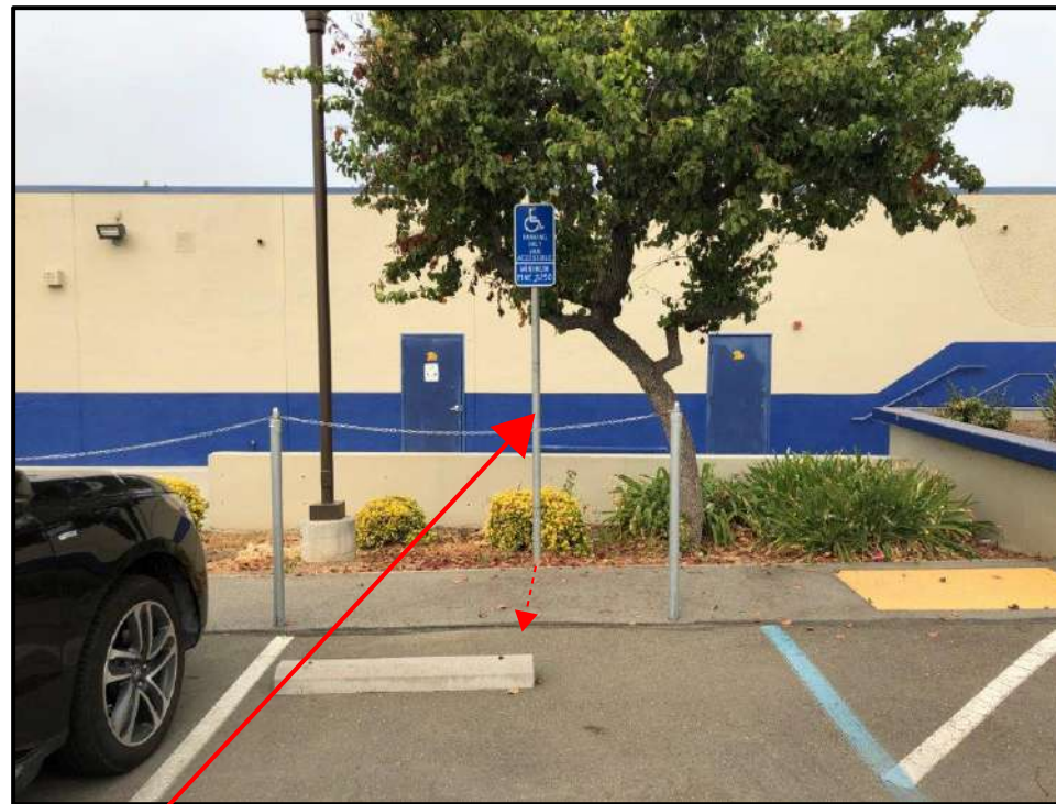
Photo 6: Relocate existing ADA parking sign and install new pole to be centered between new fence and wheel stop. Remove existing pole, footing, and backfill.
