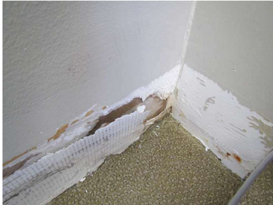
Water-damaged/mold growth on GW in SWB office, note rusted stud
