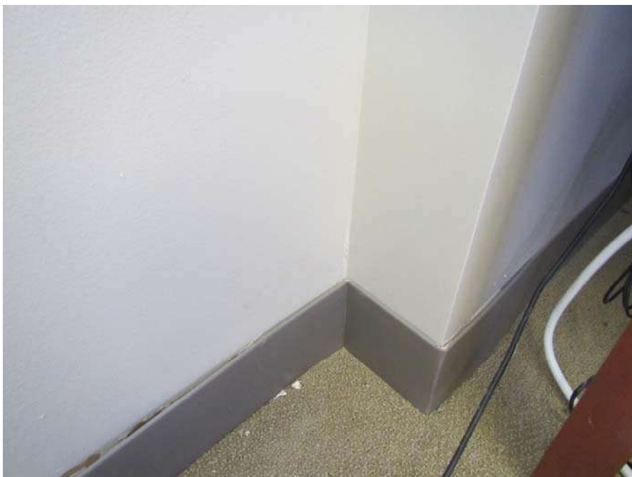
Water-damaged corner wall in SWB office
