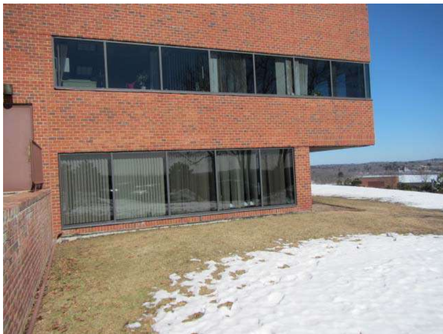
Offices experiencing water damage are located on a south-facing wall not protected by an overhang
