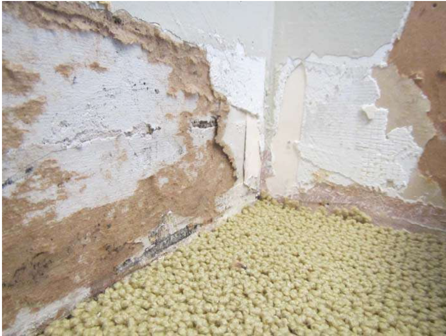
GW behind coving in JR office, note black staining indicative of mold growth
