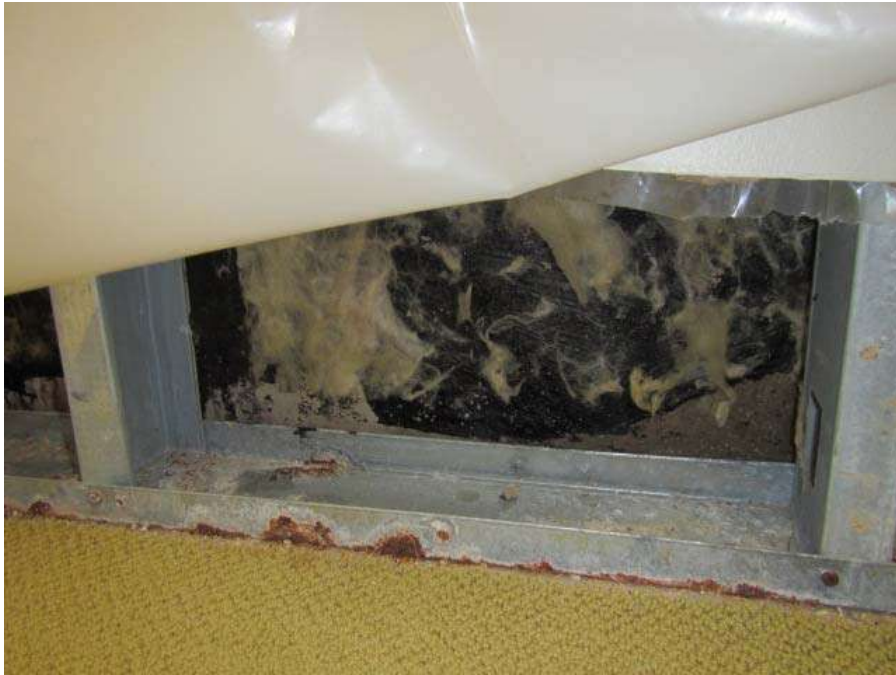
GW removed from JR office, note rust on metal frame and studs
