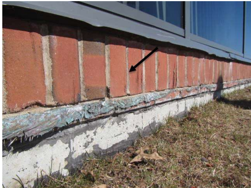
Weep holes approximately at the brick wall/foundation junction; also note damage to waterproof coating at foundation
