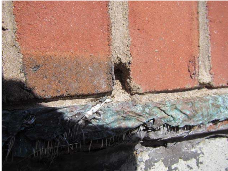
Weep holes blocked with cement or accumulated sediment from bricks/mortar
