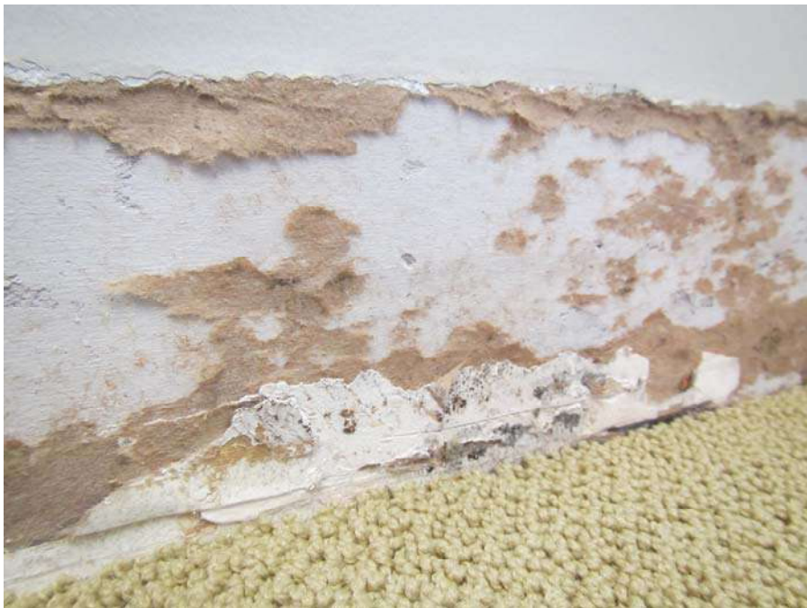
GW behind coving in JR office, note black staining, indicative of mold growth
