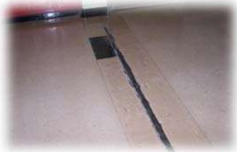
Sealed asbestos under tiles
