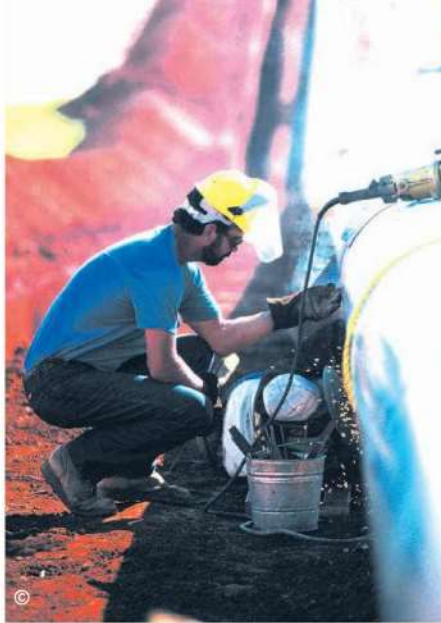
FIGURE 4 Natural Gas Pipelines More than 2,500,000 kilometers of natural gas pipelines run underground in the United States. Here, a technician prepares a new section of pipe.
