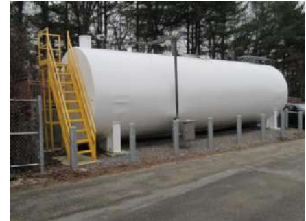
20,000 gallon oil tank located at NHS
