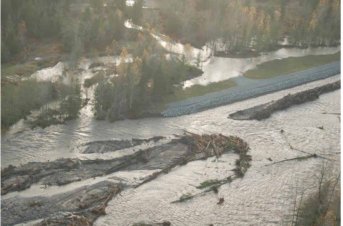
Figure 16: A Compromised Levee at Neadham Road, 2008
