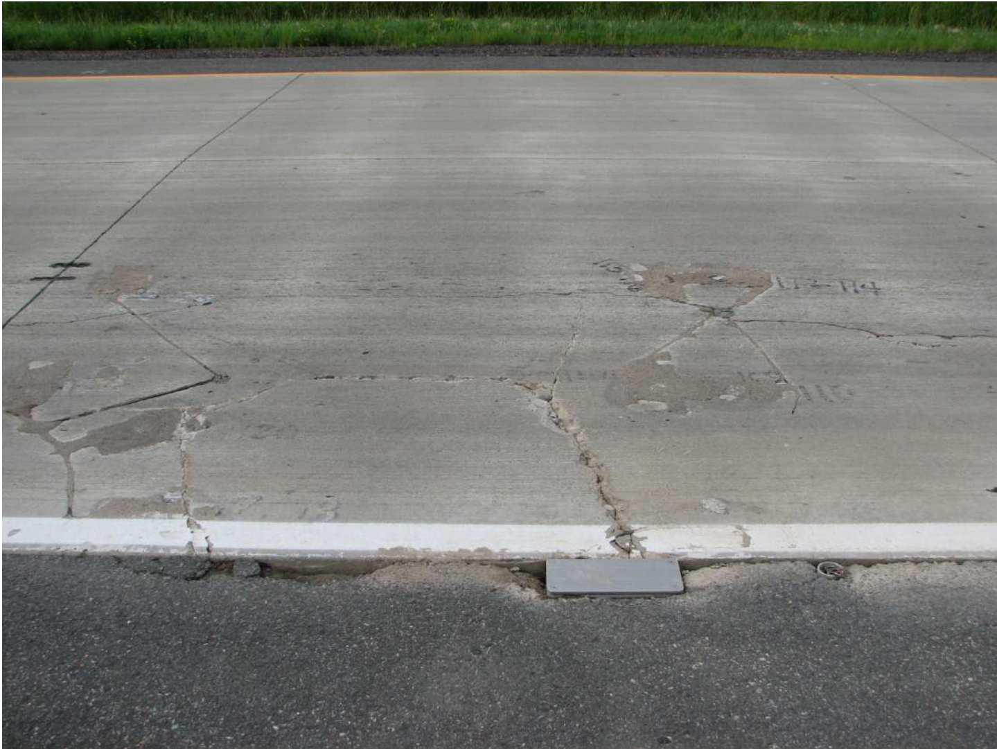
Cell 113 cracks in sensor area, July 2011
