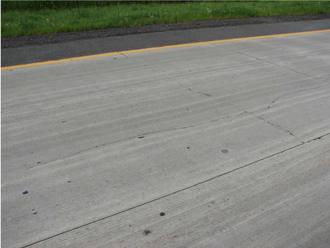
Cell 213 passing lane cracks, July 2011
