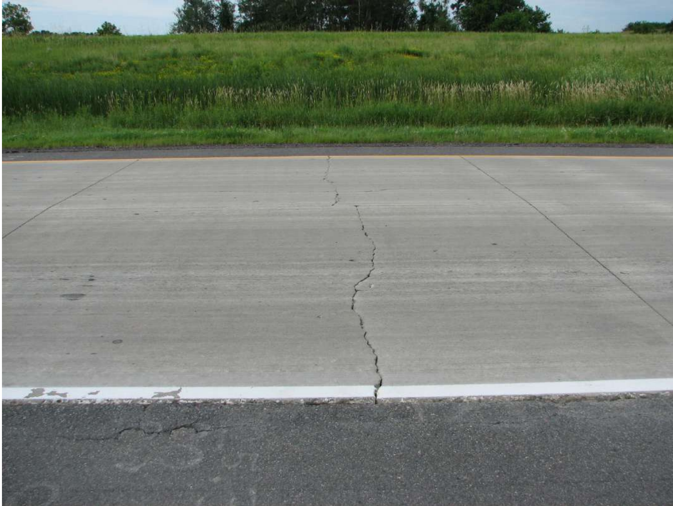
Cell 213 transverse crack, Oct 2011
