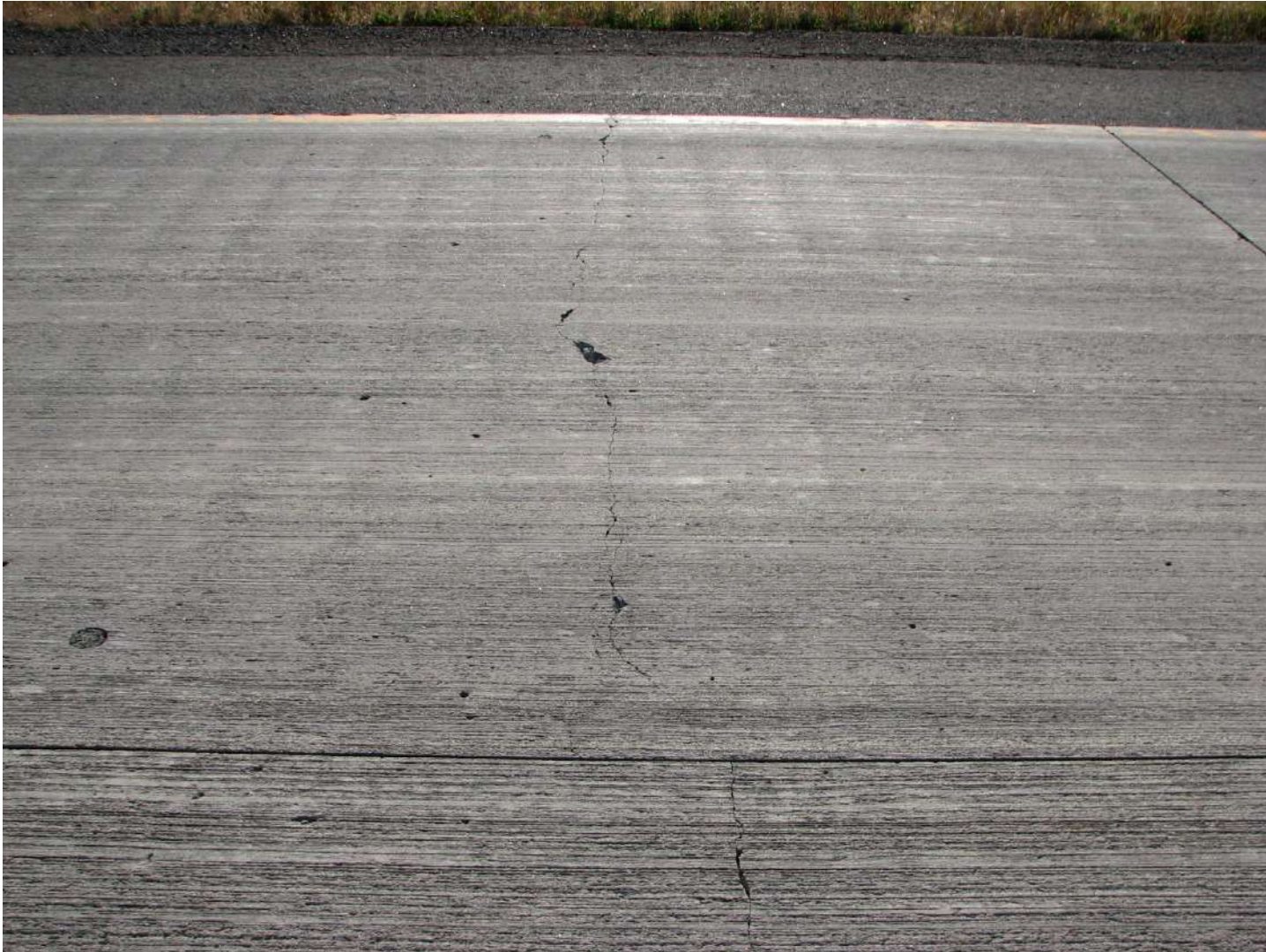
Cell 213 transverse crack, Oct 2010
