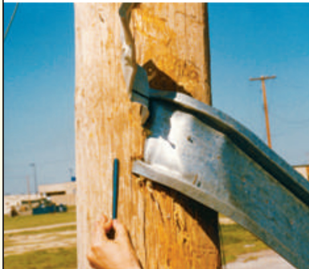
Figure 1 Tornado Damage in Kansas The force of the wind during a tornado was strong enough to drive a piece of metal into the utility pole.
