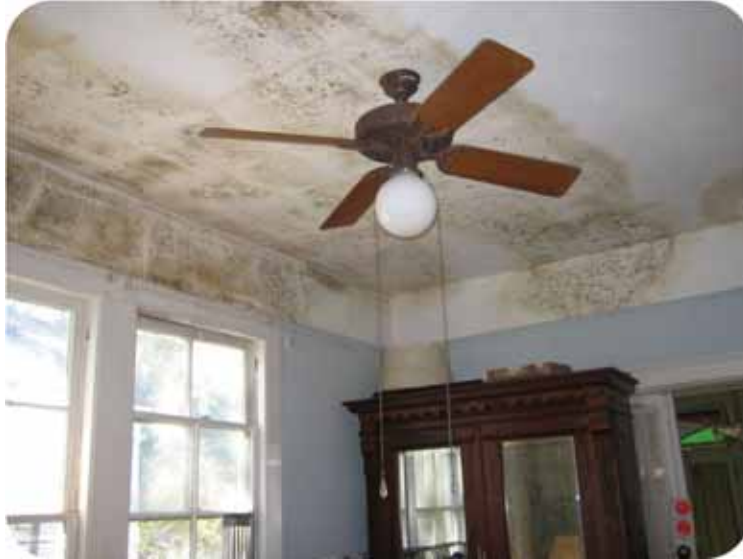
Figure 14.28: The mold growing on the walls and ceiling of this storm-damaged home may be harmful to human health.
