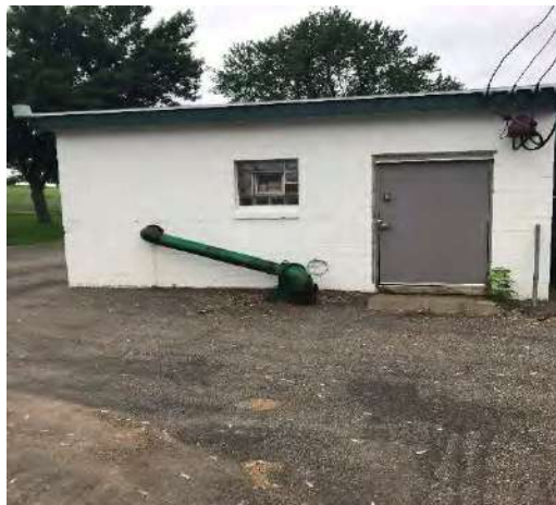
Older deep well pump in good condition
