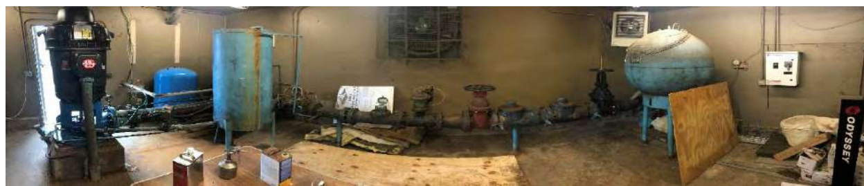
Below – Older Pump House and Controls
