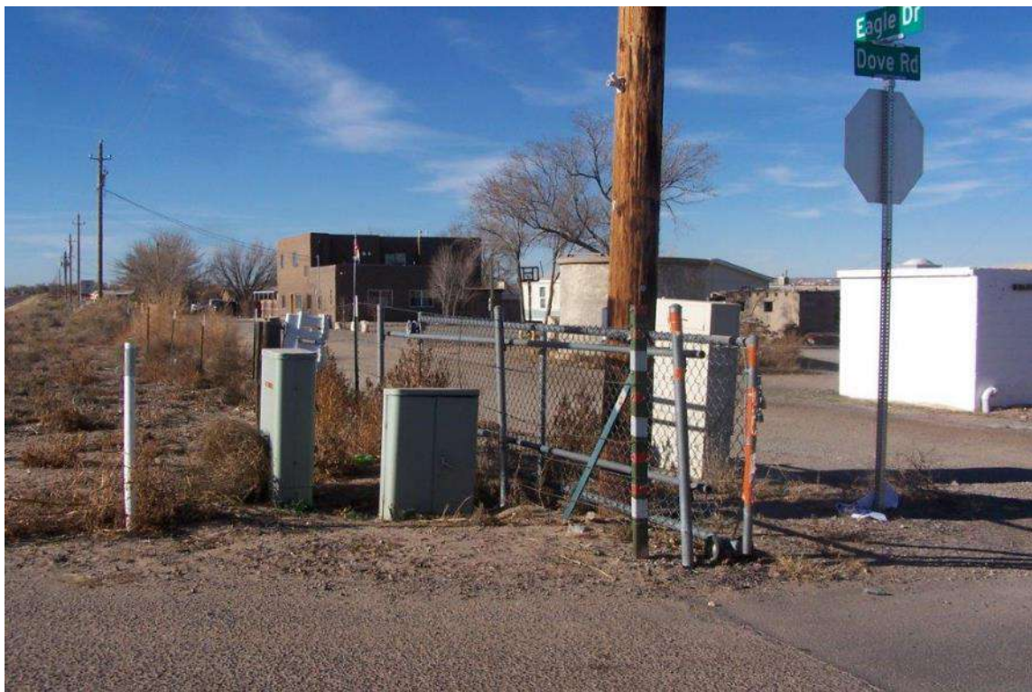
Figure 50: Reservation Area Copper Telephone Infrastructure
