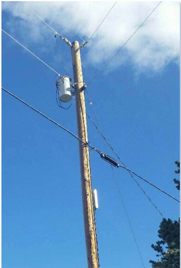
Figure 43: Old Santa Fe Trail – Poles with Ample Space for Broadband Attachment
