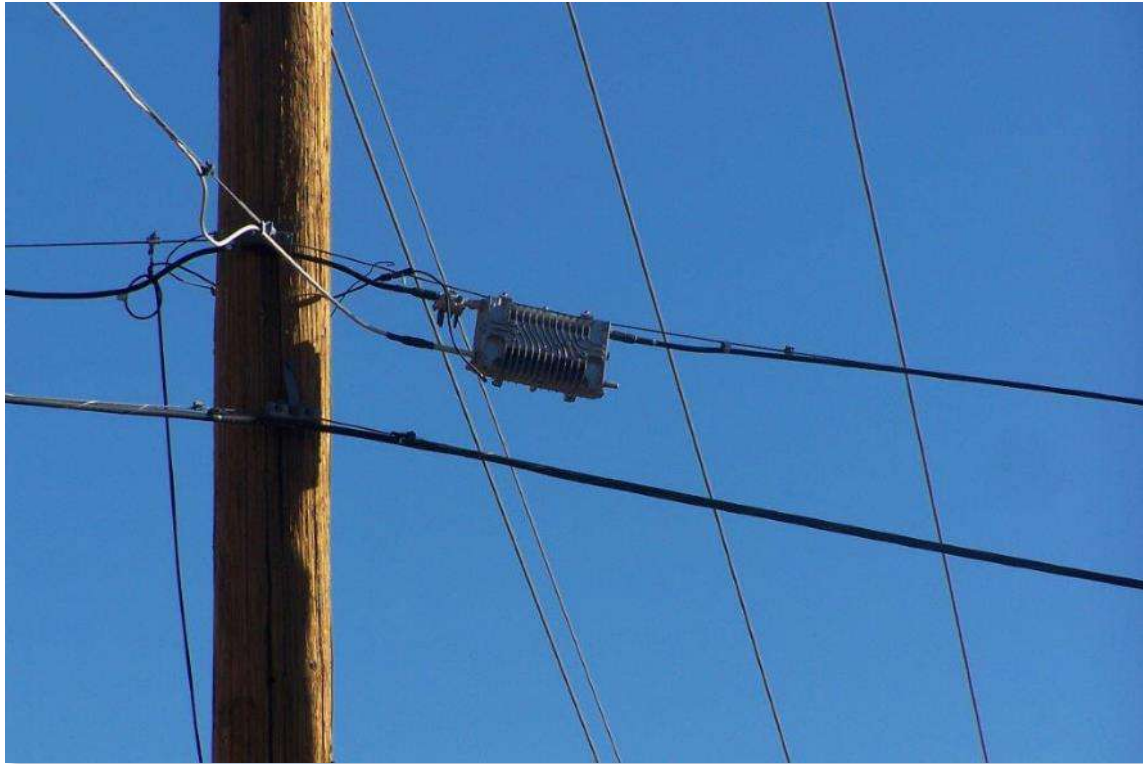
Figure 49: Reservation Area CATV Infrastructure
