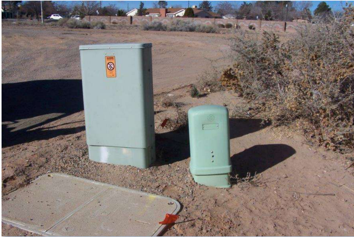
Figure 48: Rio Rancho Buried Telephone Infrastructure
