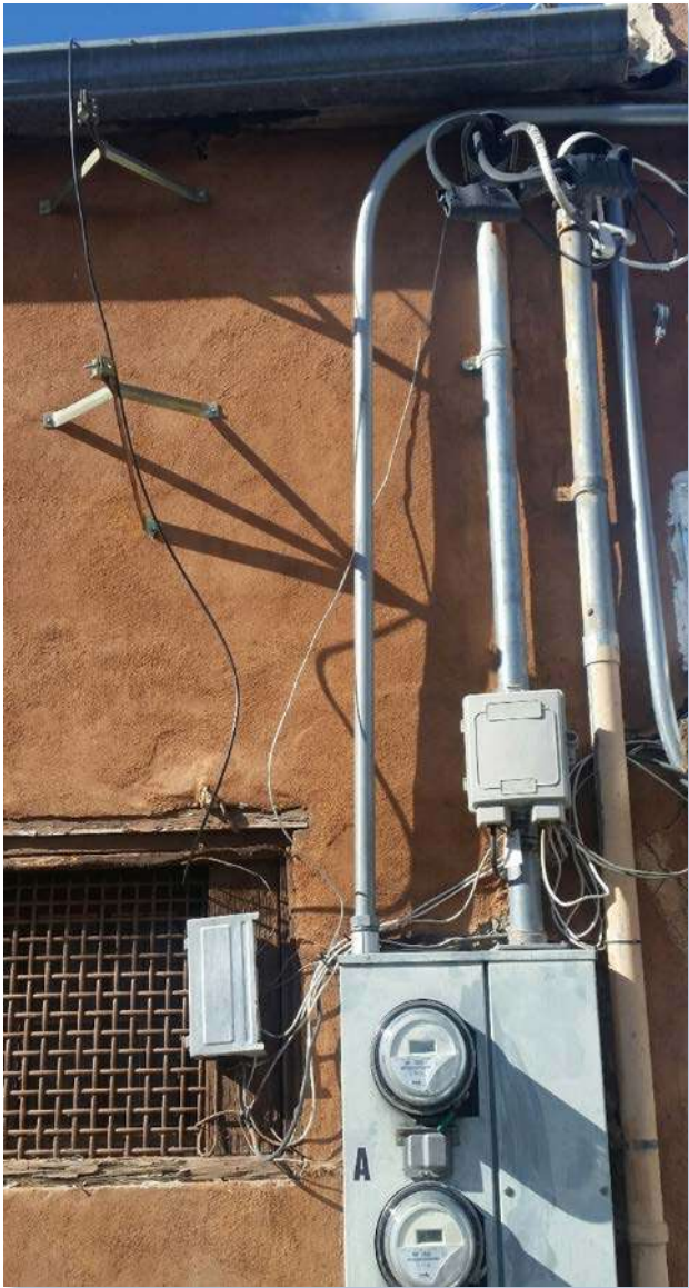
Figure 39: Downtown Santa Fe – Assorted Cables to Rooftop
