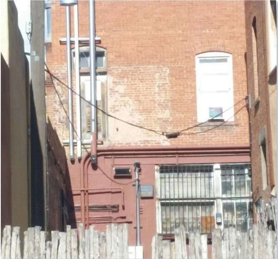
Figure 40: Downtown Santa Fe – Ad Hoc Telecommunications Cabling Hanging from Building to Building
